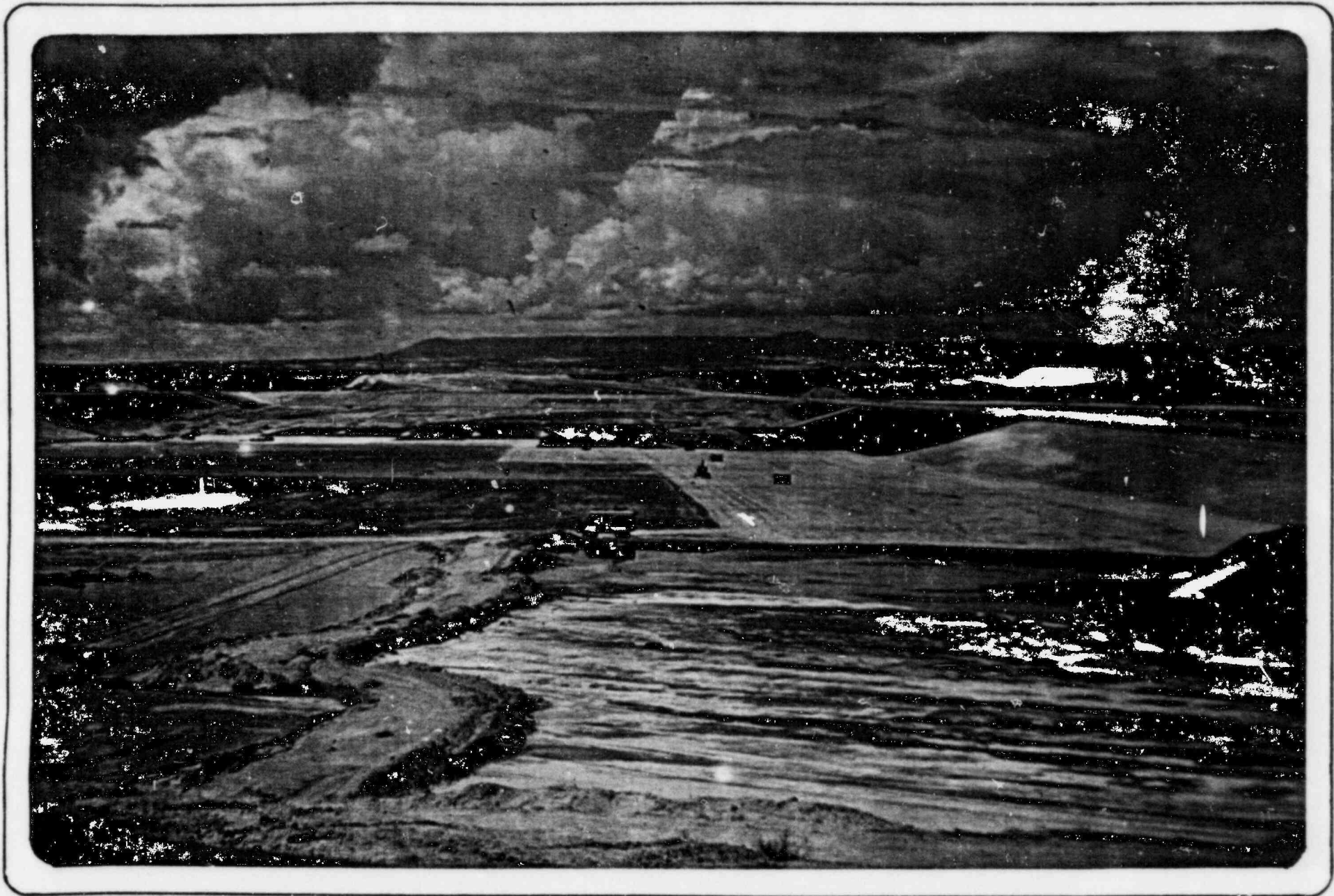
Cell 3 - Liner Installation, approximately 50% complete. (Note storage area for dewatered tailings sands - lower right)
