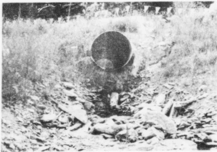
Figure A-29. Downstream sedimentation study rod at Station 8, 10 August 1981. No noticeable sediment accumulation since May, but ditch appeared deeper.
