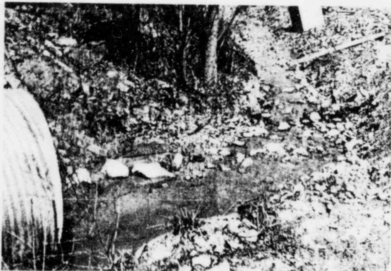
Figure A-27. Downstream sedimentation study site at Station 8, 27 March 1980. Study rod was removed by significant construction activity and temporary alteration of stream flow direction.
