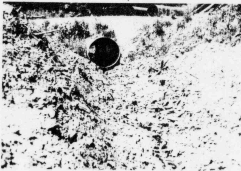
Figure A-28. Downstream sedimentation study site at Station 8, 29 May 1980. New study rod placed in March was again removed by continuing construction activity. No sediment accumulation was observed. Study rod was not replaced.
