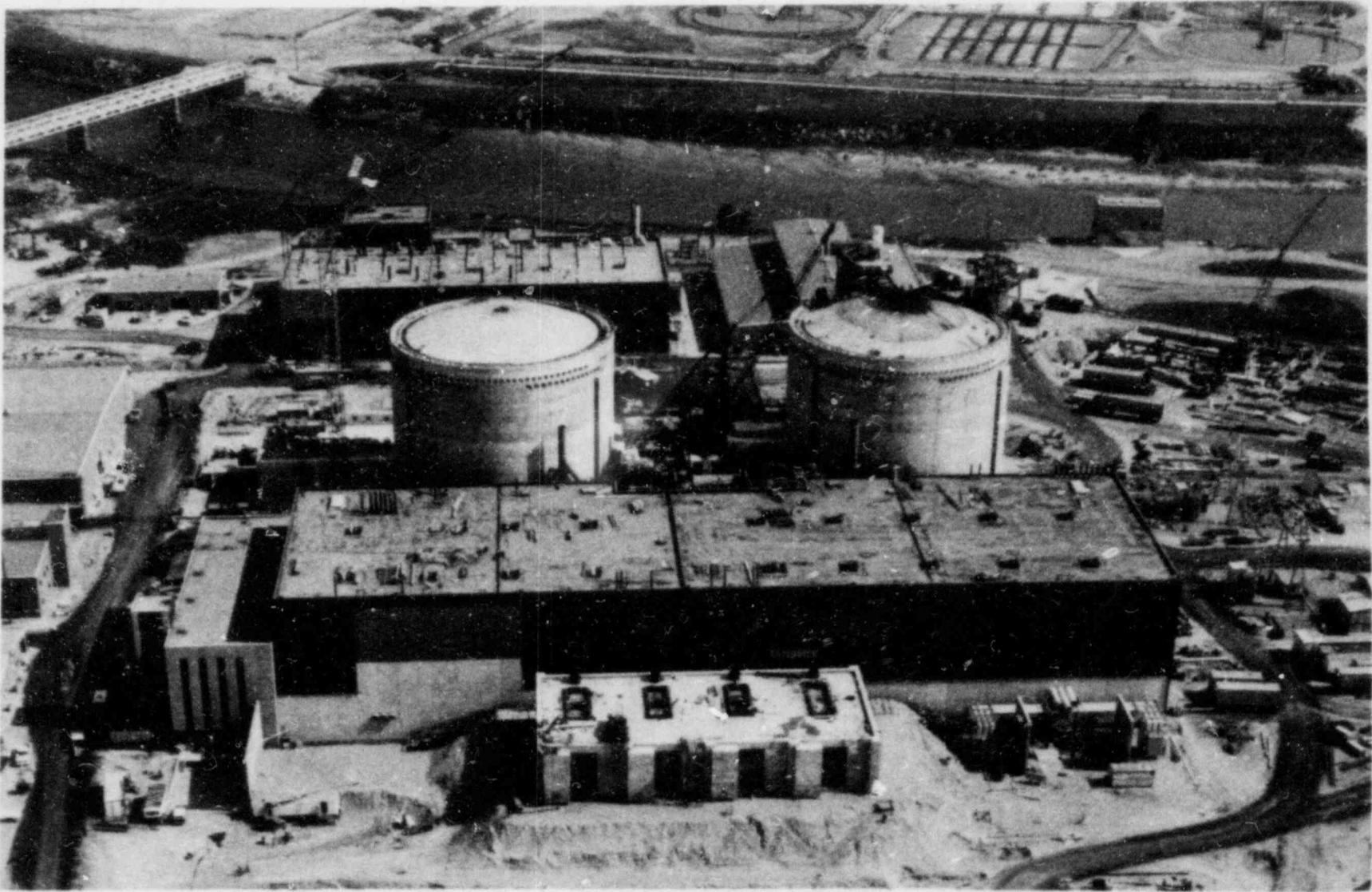
Figure 2.10 Photograph of Midland Plant showing 20-ft sand surcharge for DGB in place in mid-1979
