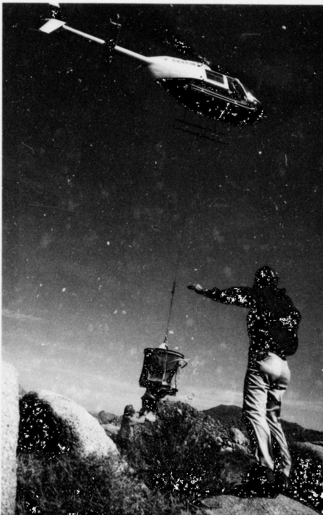
Helicopters are being used to transport men and materials, such as concrete for transmission tower bases, to construction sites along the Southwest Powerlink.
