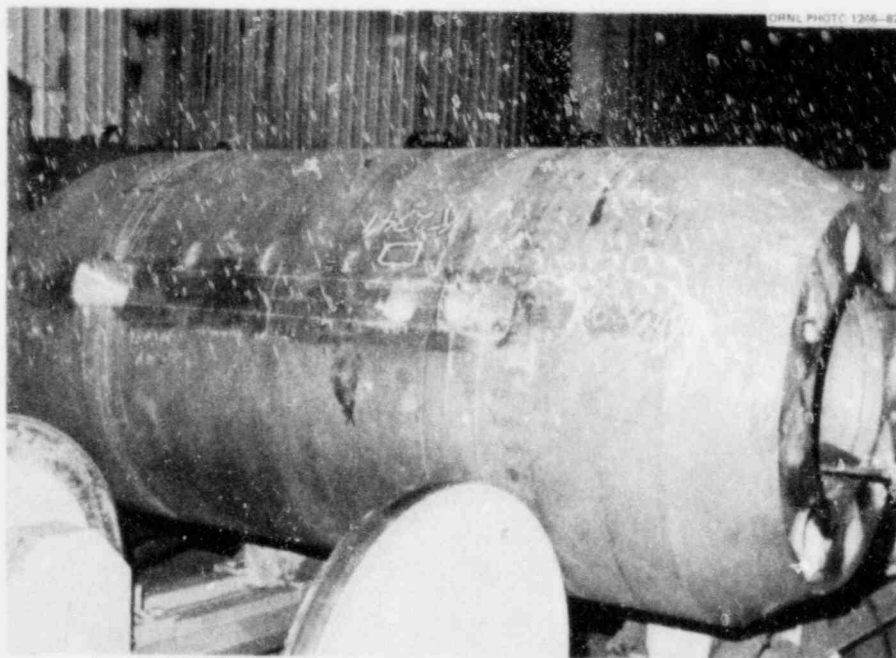
Figure 24 Completed Submerged-Arc (SA) Portion of the Seam Test Weld and Manual Metal Arc (MMA) Weld Cavities of the Vessel
