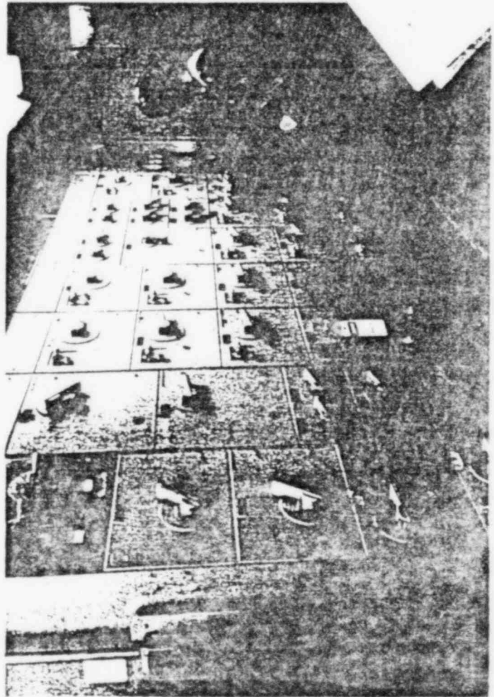
Unitrol Motor Control Centers
