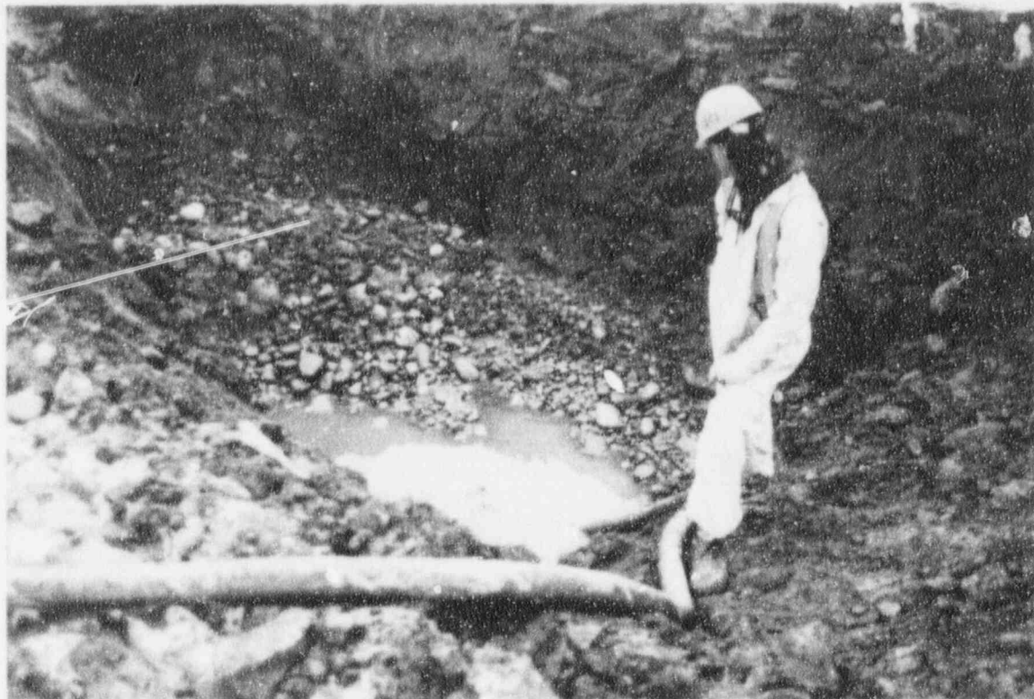
TP M-CF-25. Unsuccessful attempt to dewater the pit to allow collection of samples below the water table.
