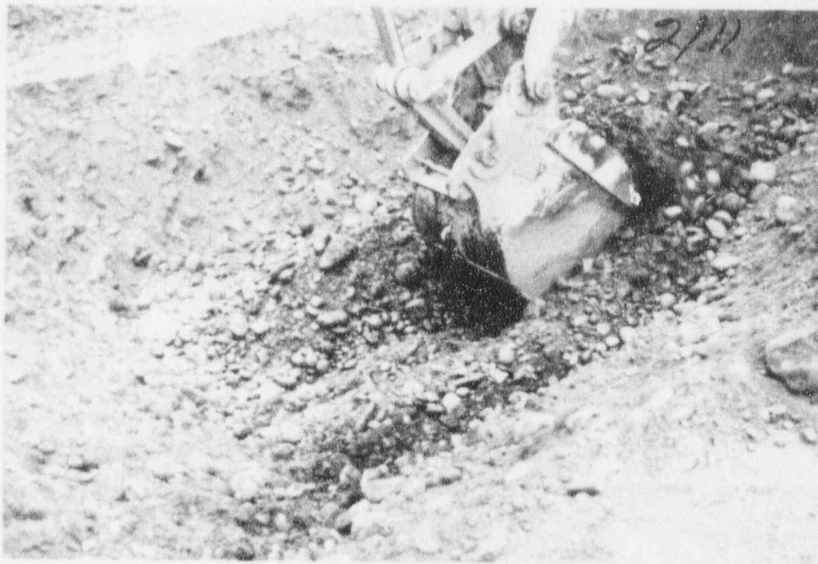
TP M-CF-22. About 4-feet of road fill overlying the in-situ cobbles and gravels.
