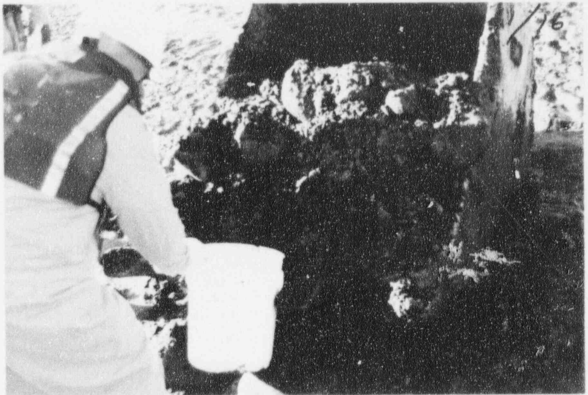
Gravel samples were collected in one-foot intervals and placed on plastic sheets in order to carry out the gradation analysis.
