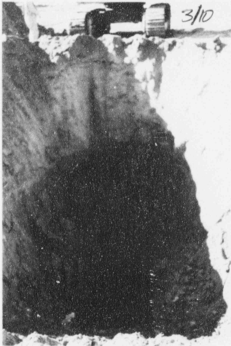
TP M-CF-07. Tailings overlying clay soil and gravels. Perched water in the tailings and equipment vibration caused severe caving of the tailings resulting in contamination of samples from the underlying material.
