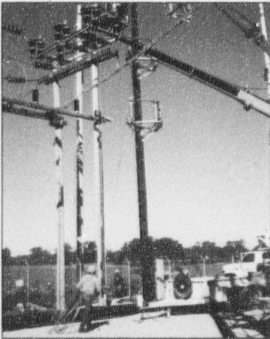
As part of CIPCO's program to improve service reliability, motor-operated switches are being installed across the system. Above, Wilton crews work to complete the '93 project.
