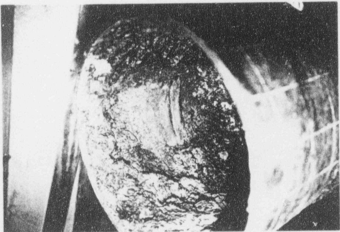
Supply to RHR Heat Exchanger
