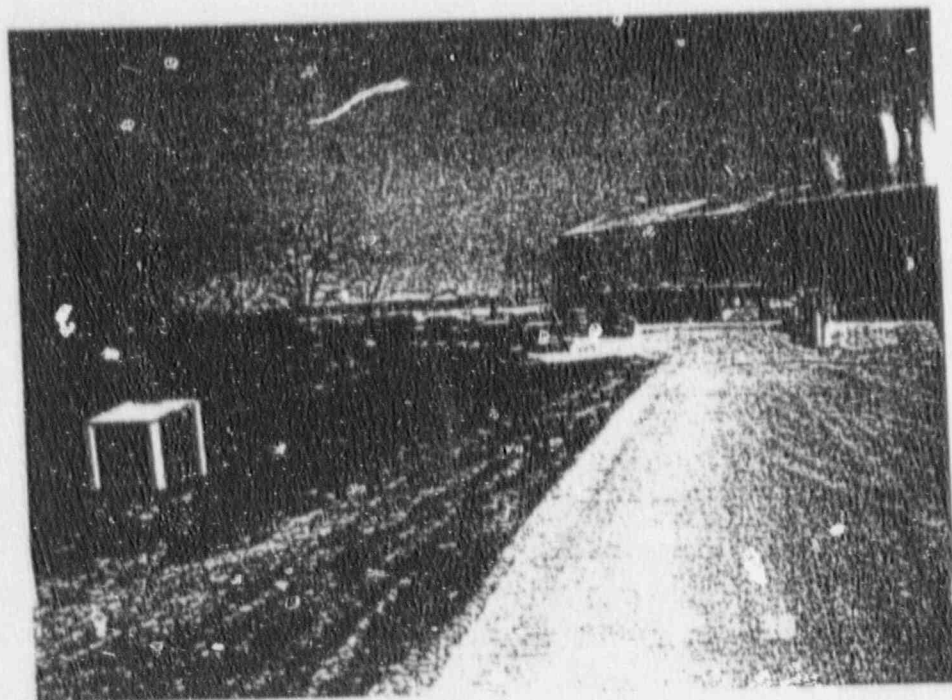
PHOTO:10 PCS# 2593 ROLL/PICTURE: 3/16 SITE NAME: SHIELDALLOY METALLURGICAL DESCRIPTION: DUST CLOUD GENERATED FROM HEAVY EQUIPMENT OPERATION ON SMC PROPERTY. DATE/TIME: 4-18-90 / 1236 PHOTOGRAPHER: NALSCH FILM: 35MM, 200 ASA, NO ATTACHMENTS
