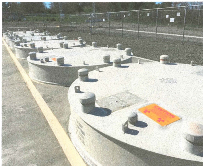
Figure 4 - Picture of HB ISFSI installed vault lids
