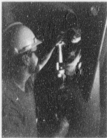
INPO assistance visits may focus on a specific area such as proper maintenance of a plant component, or some other important aspect of overall nuclear plant operations. Here, mechanics at Susquehanna align a condensate pump.
