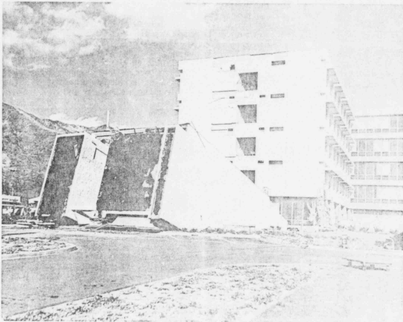
OLIVE VIEW HOSPITAL FOLLOWING THE SAN FERNANDO EARTHQUAKE OF FEBRUARY 9, 1971 (Recommendation No. 7)
