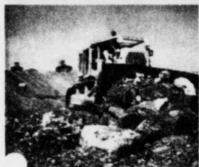
Bulldozers work to restore mined land to its original contour near La Cygne Station.
