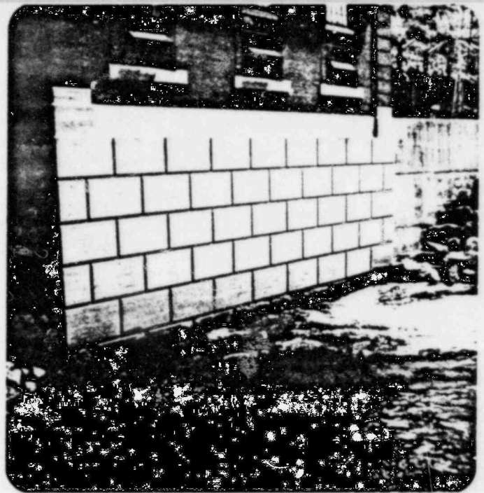
Photo No. 6 Face of Powerhouse Over Draft Tubes Note Deteriorated Concrete at Water Line
