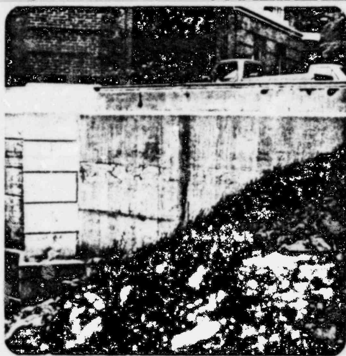
Photo No. 6 Retaining Wall Adjacent to Powerhouse Note Cracking and Staining
