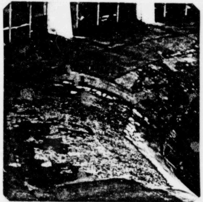
Photo No. 4 Interior Slope of Glory Hole Spillway Note Spalled Concrete
