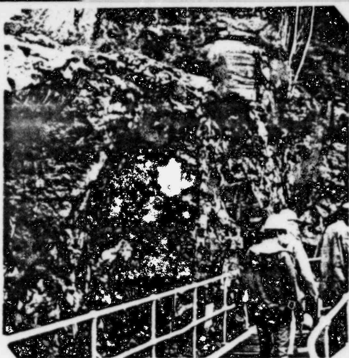
Photo No. 5 Fractured Rock Face at Intake Note Overhang and Jointing
