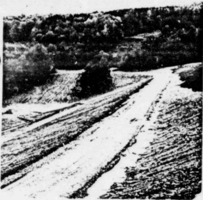
Photo No. 1 View Across Dam at Top of Berm Note Minor Erosion and Ponded Water, Sediment Collection at Toe of Dam. 1981 Modification
