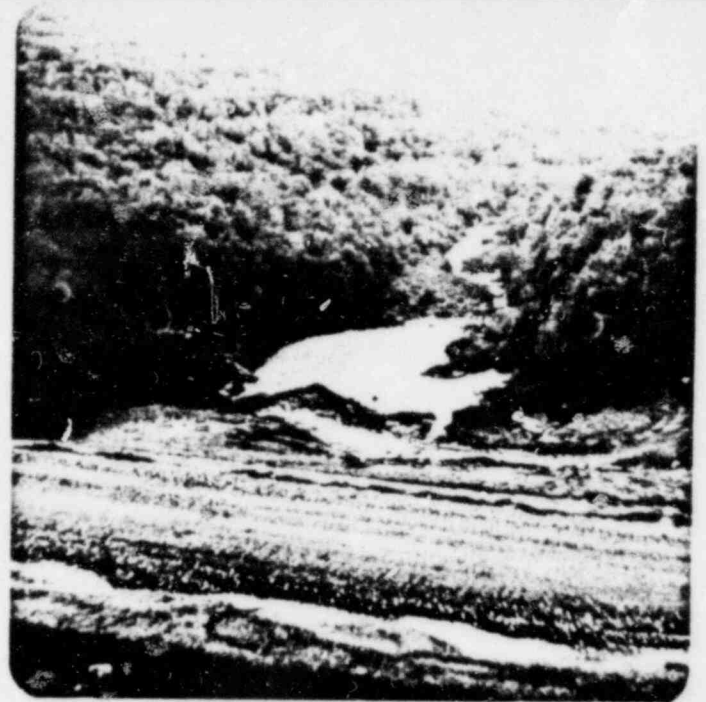
Photo No. 2 View of Downstream Slope at Dam Centerline. 1981 Modification. Note Eroded Material and Cloudy Water at Toe of Dam
