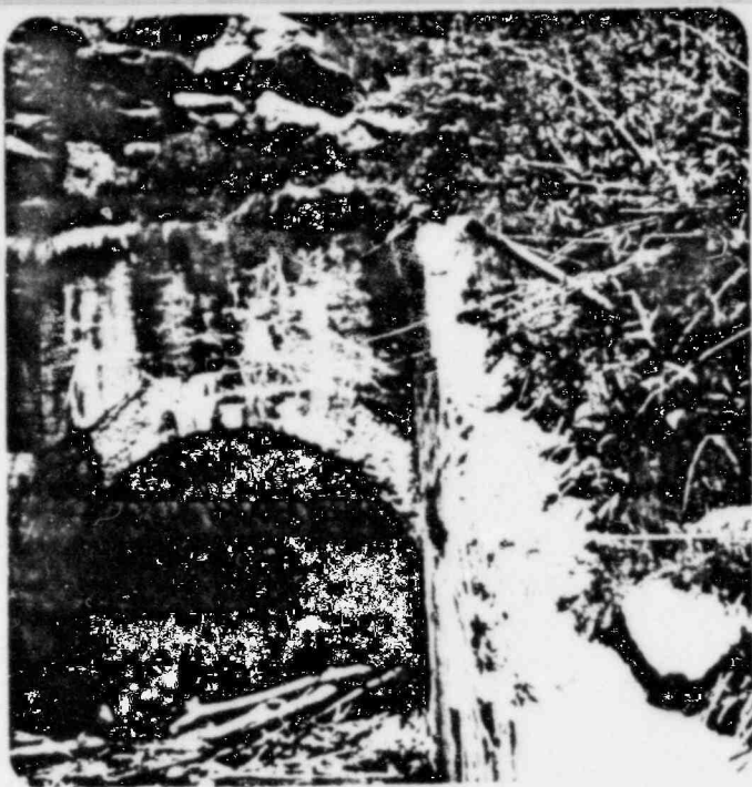
Photo No. 5 Downstream End of Diversion Tunnel Note Deteriorated Concrete, Debris
