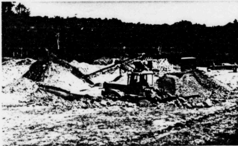
PHOTO 2 "CARBIDE PIT" — FILTER BLANKET BORROW SOURCE. MATERIAL PROCESSING INCLUDED SCREENING AND CRUSHING (8-20-81)
