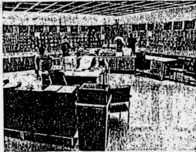
This is the control room at the Vermont Yankee nuclear power plant.
