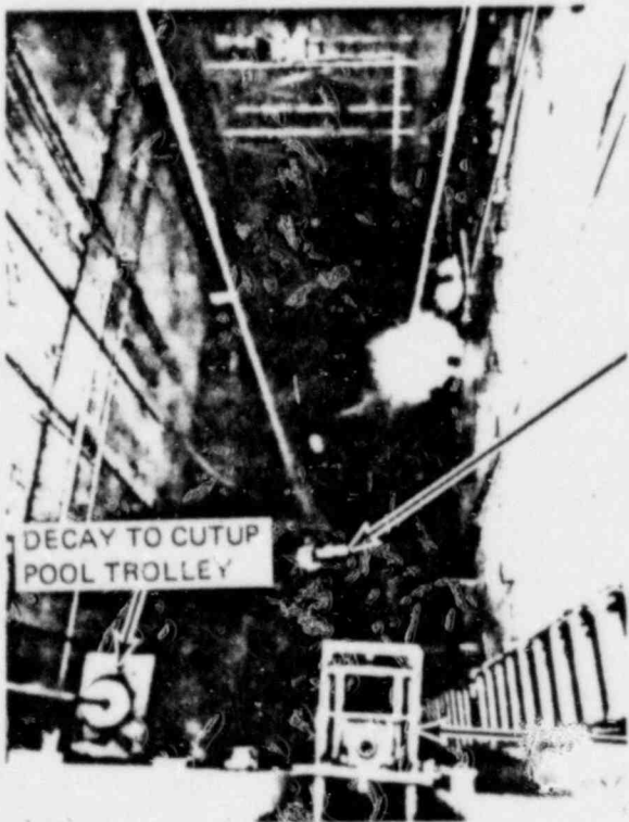
BELLOWS PUMP HANGING ABOVE WATER SURFACE
