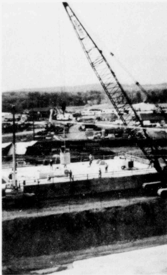
Removal from waste storage of a liner from the first stage of EPICOR-II for shipment to the Battelle Columbus Laboratories for examination.
