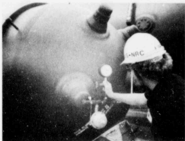
An NRC inspector examines a gauge atop a pressurizer in a storage area at Marble Hill (Ind.) nuclear power plant.
