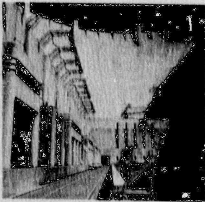
Upgrading of the units at Hoover Power Plant will result in additional capacity entitlements to six SCPPA members.
