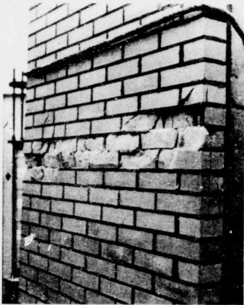
FIG. 3.13 TYPICAL FAILURE OF BRICK WALLS WITH HIGH VERTICAL COMPRESSIVE LOADS
