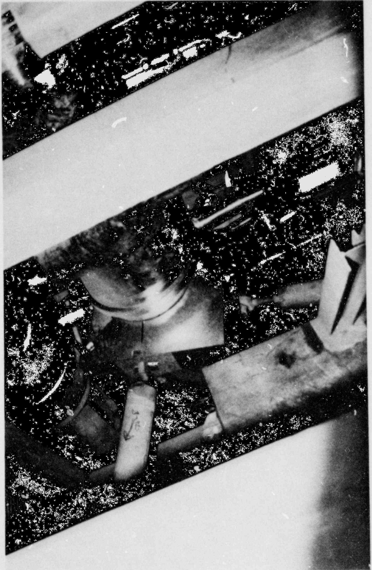
Kuosheng Recirc Control Valve B and Pipe Supports
