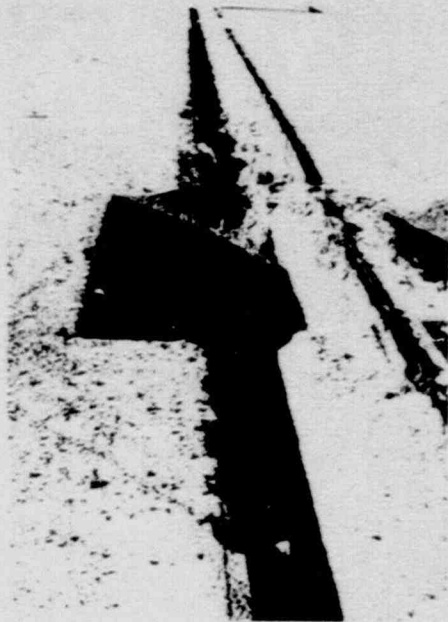
Looking west across the south sump and down the drain line in the concrete slab. (Frame 1, Roll 469609)
