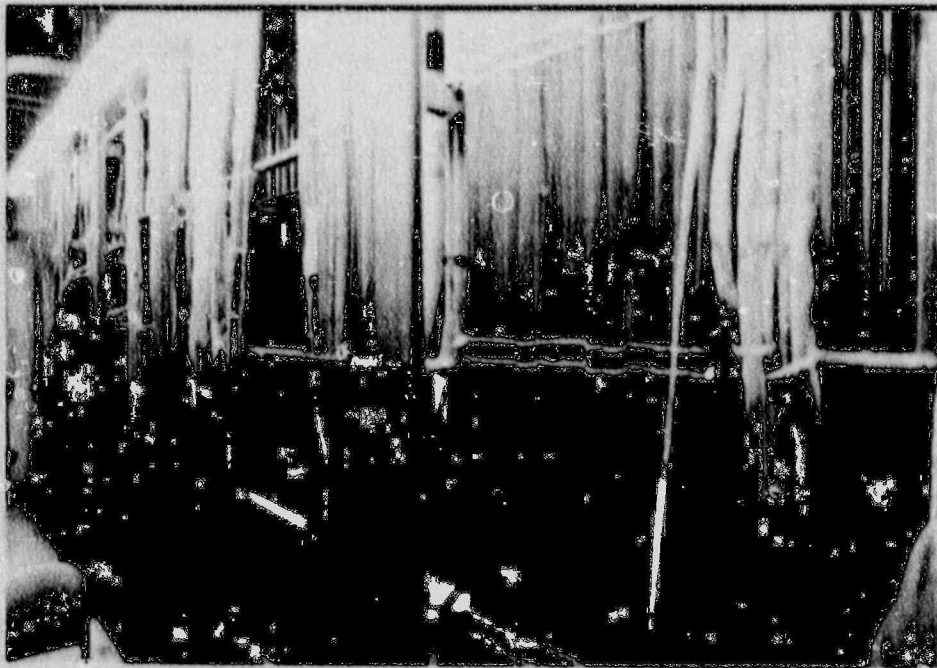
FIGURE 10. Electrical Cable from Radiation (Top) and Control (Bottom) Areas for NPAR Studies at INEL
