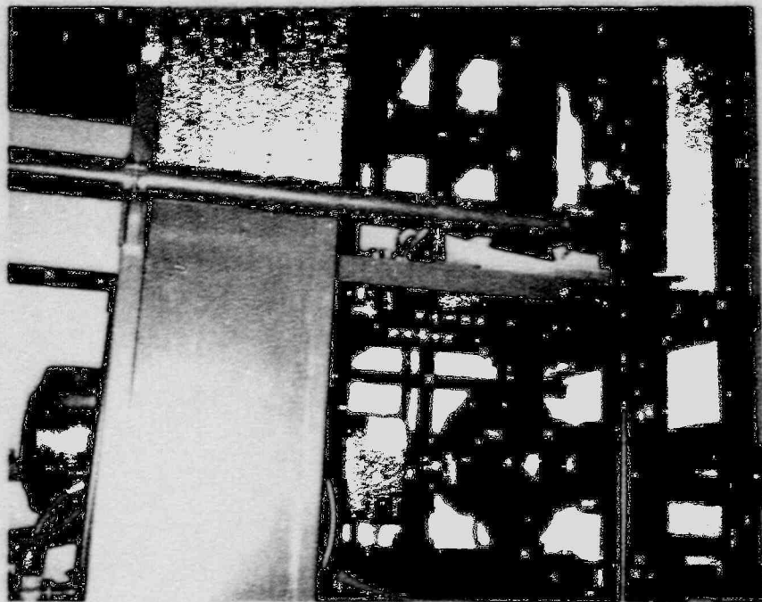
MAIN CIRCULATING PROCESS PUMP
