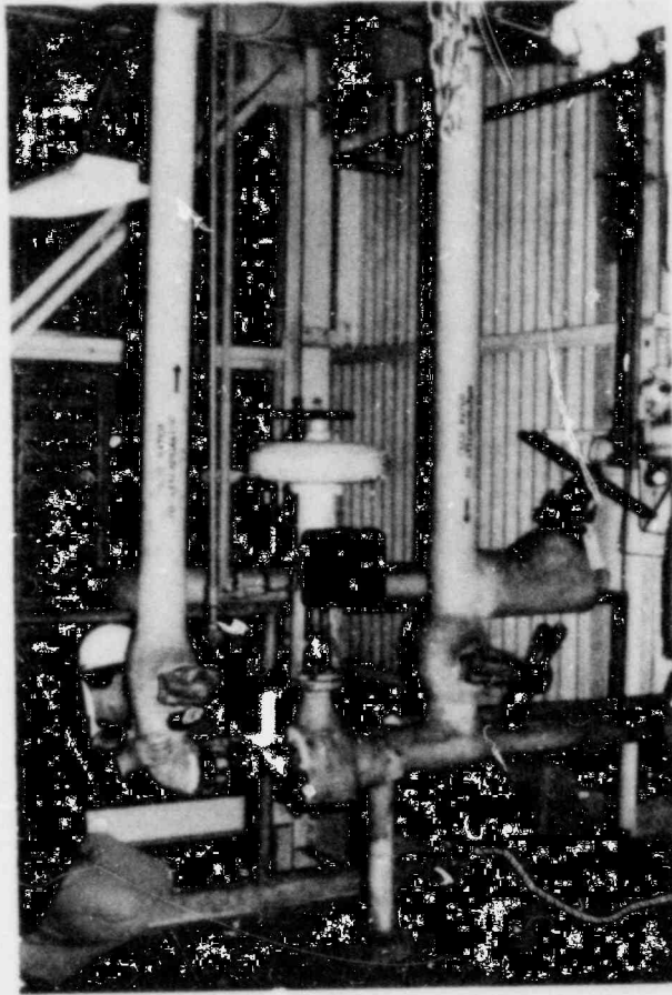
Figure 14: Eroded 2-in. Spool Piece of the Unit 1 Boiler Feedwater Piping Which Leaked at a Weld. (Note the chipped grout under the left side of the support base plate at floor.)
