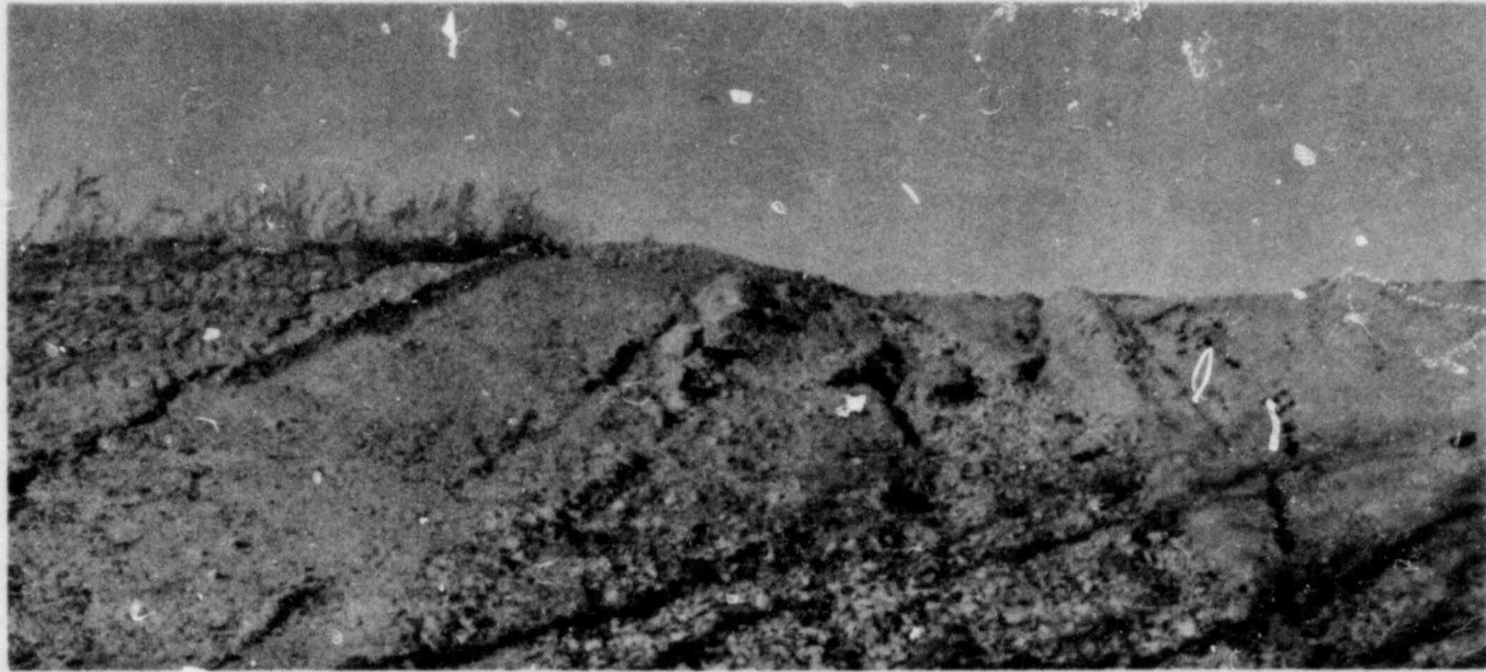
SLOPE AT SOUTH END OF SITE LOOKING NORTH FIGURE 9 - SURFACE WATER SWALE - NOVEMBER 5, 1980
