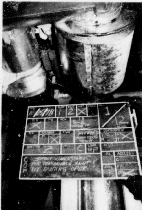
Figure A.27 Hydraulic snubber (note inaccessibility)
