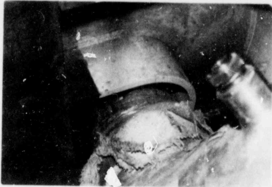
Figure A.11 Pipe whip restraint, weld inaccessible for inservice inspection
