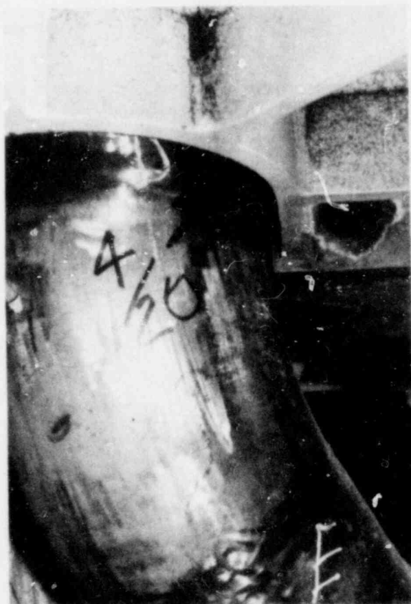
Figure A.10 Pipe whip restraint, weld inaccessible for inservice inspection
