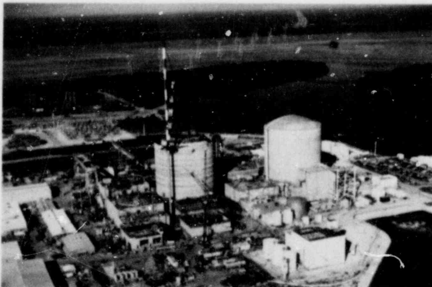
This aerial photo of the St. Lucie Nuclear Power Station in Florida shows the reconstructed derrick which was blown down by Hurricane David in September 1979. Two buildings under construction as part of Unit 2 of the plant were damaged by the derrick's collapse. Unit 1, at right, has been in commercial operation since 1976.
