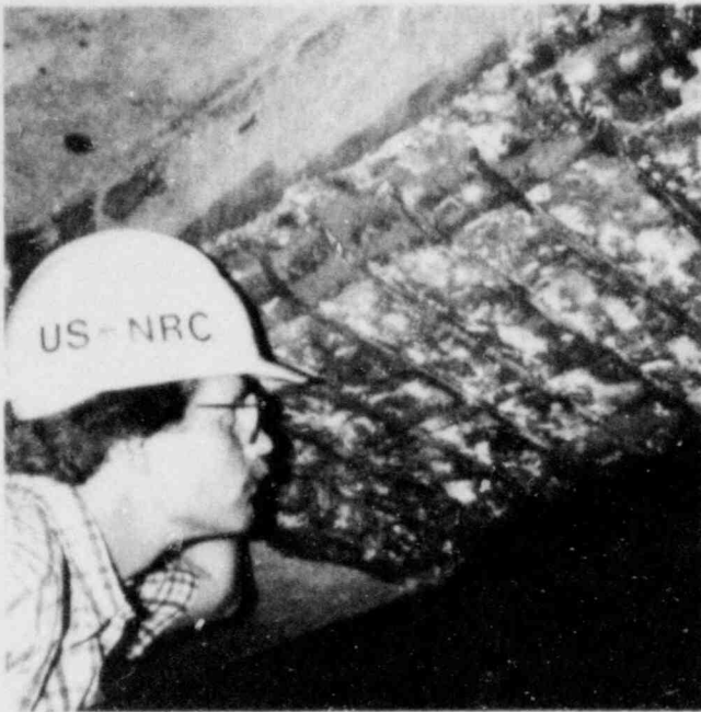
NRC inspector examines "honeycombing" in containment concrete at the Marble Hill Nuclear Power Station, under construction in Indiana. Continuing construction deficiency problems led to a show cause order by NRC's Office of Inspection and Enforcement and corrective actions. (See Chapter 9 under "Investigations.")
