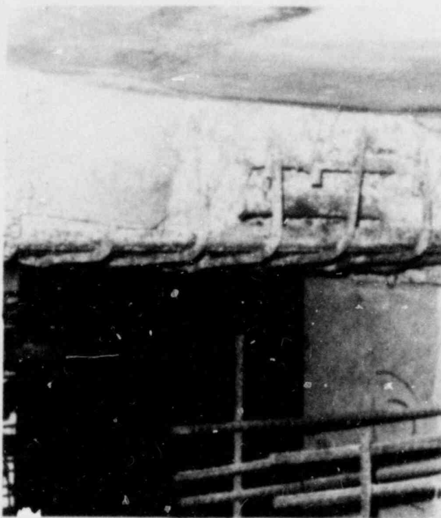
"Honeycombing" in concrete at the Marble Hill Nuclear Generating Station in Indiana was one of a number of construction deficiencies which led to an NRC-ordered suspension of work on safety-related construction for several months.
