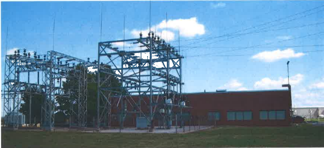
South end of Electrical Substation, with Service Building in background, from the west (9/27/2005)
