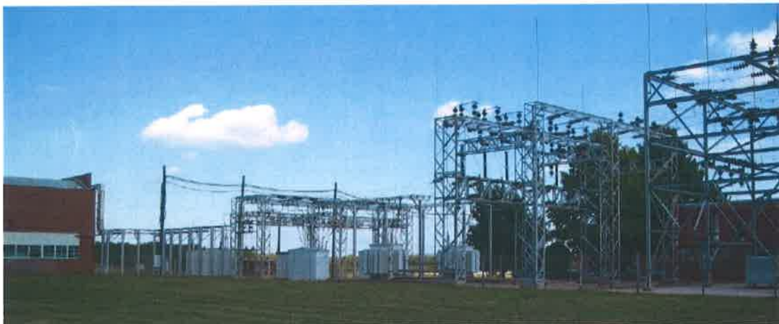
North end of Electrical Substation, with Sintering Building in background, seen from the northeast (9/27/2005)
