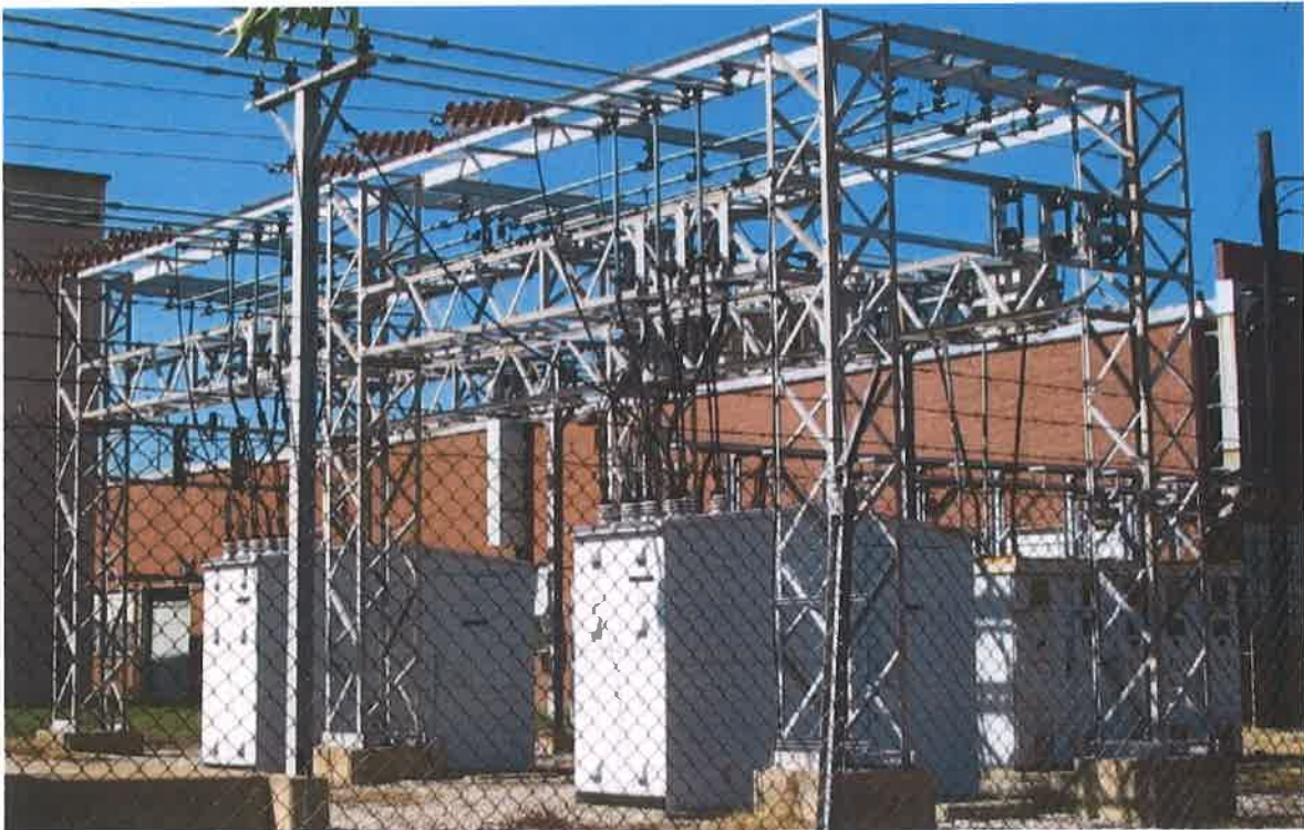
Transformer, Electrical Substation (9/27/2005)
