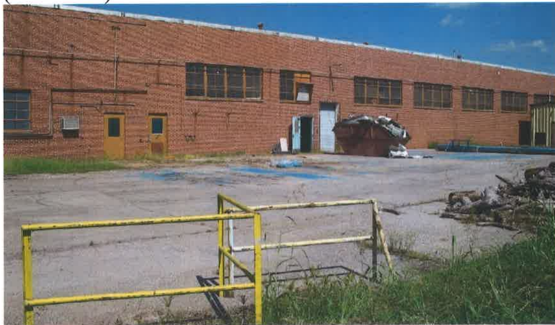
South side of Service Building, showing woodpile, paint overspray on ground, metal building and dumpster (9/27/2005)
