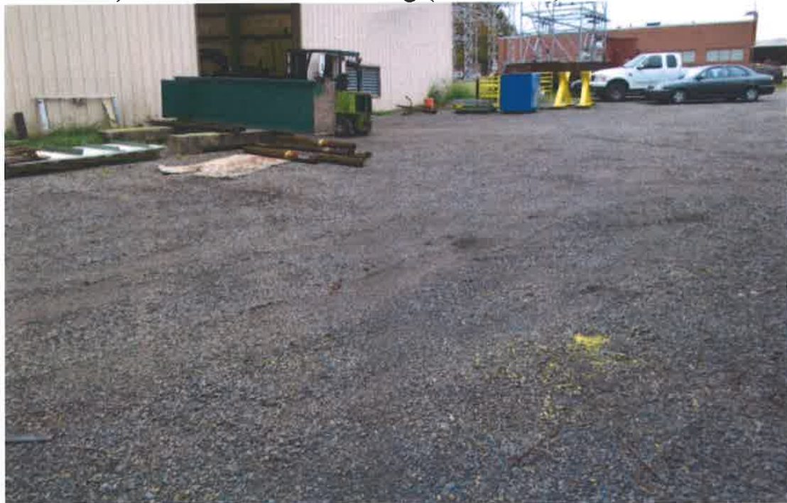
South end, Electron Beam Building, showing paint overspray on gravel parking lot (10/27/2006)
