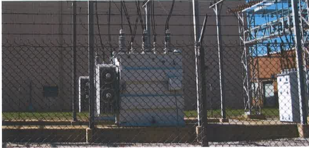
Transformer, Electrical Substation (9/27/2005)
