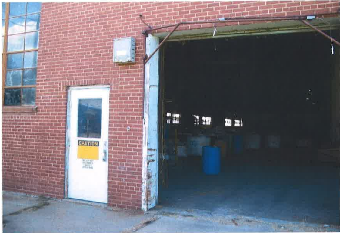
Sintering Building, east doors, showing drums and sacks of chemicals stored inside (9/27/2005, subsequently removed)
