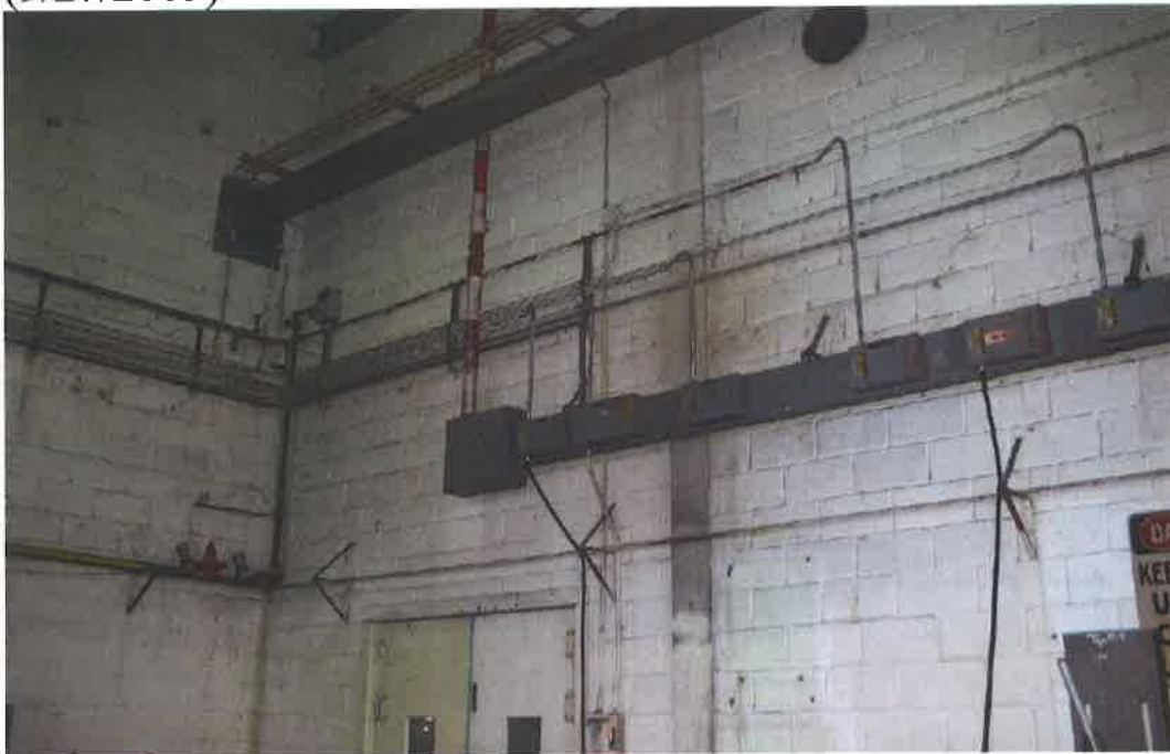
Powder still visible on upper part of walls (10/27/2006)
