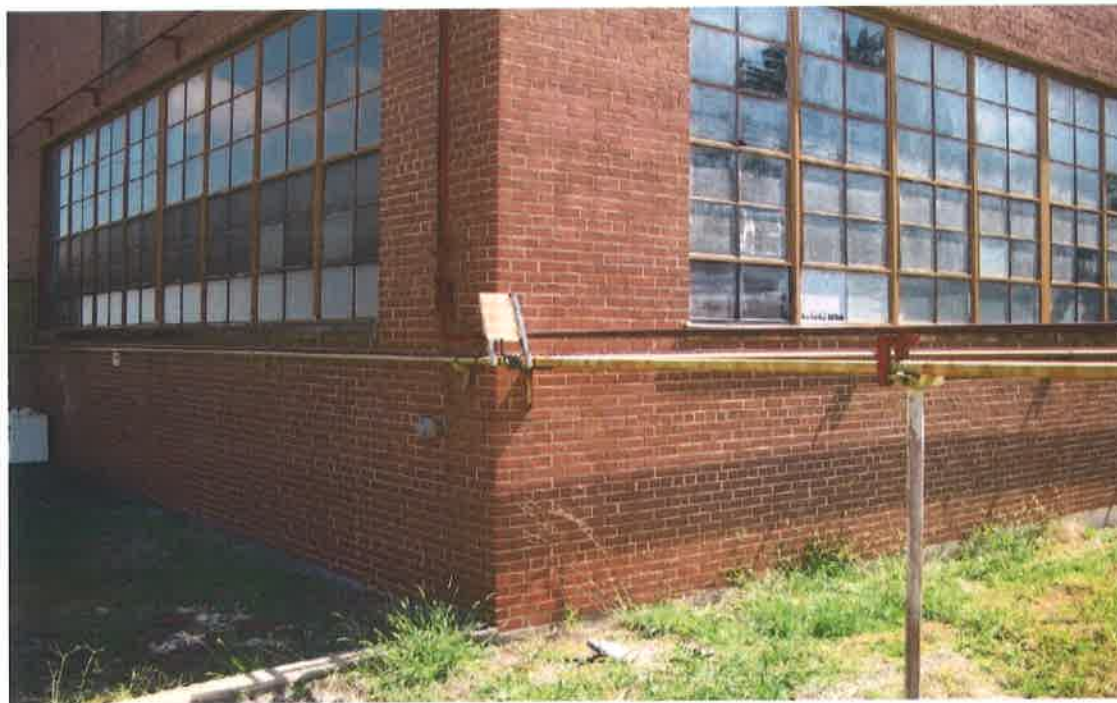
Shut-off valve on aboveground line at northwest corner of Sintering Building
