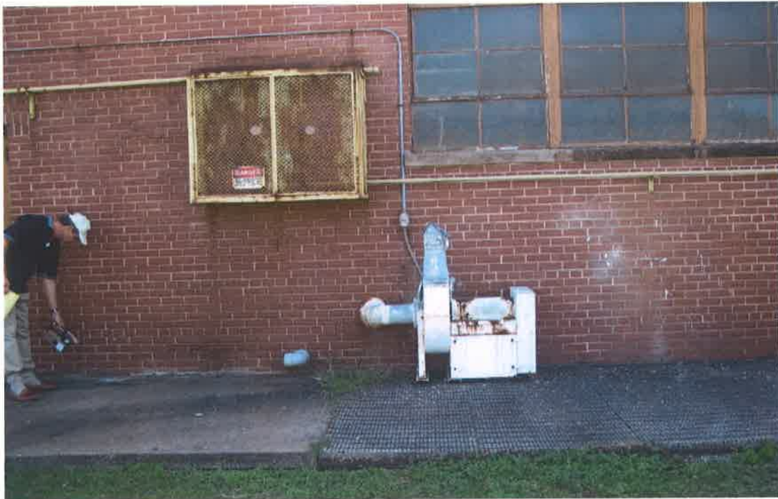
North side of Sintering Building, showing exhaust fan, valve box and possible floor drain
