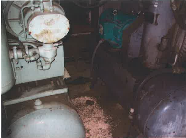
Air Compressors, spilled fluid, Building 6 (10/27/2006)
