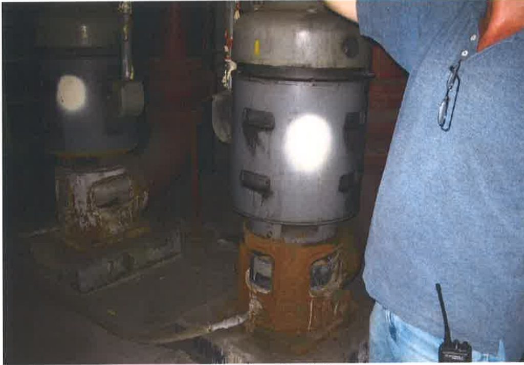
Cooling water pumps, Sintering Building (9/27/2005)
