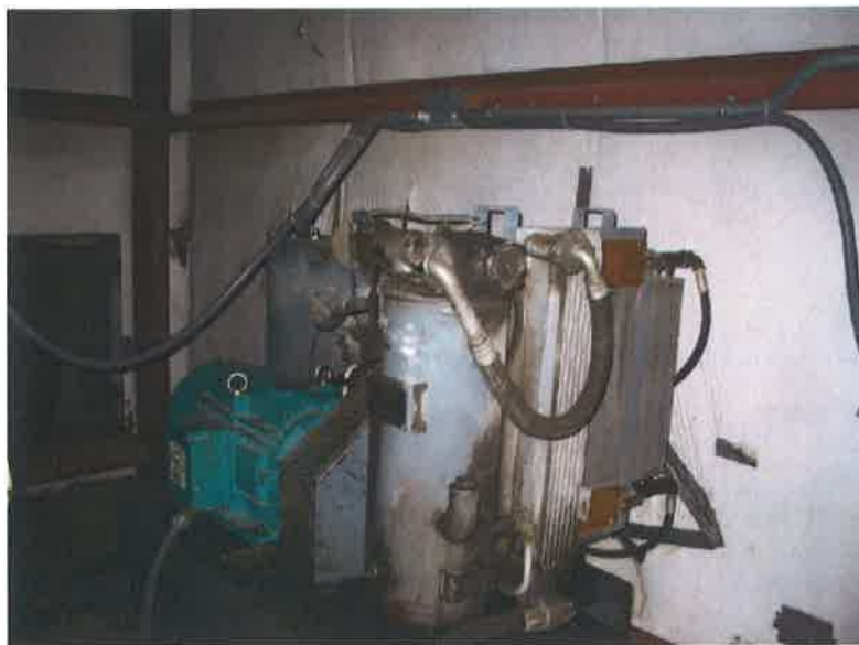
Air compressor, Building 6 (10/23/2006)
