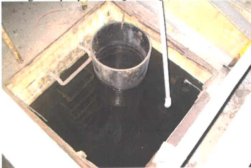
Cooling Water Reservoir with riser pipe and stanchions (10/27/2006)
