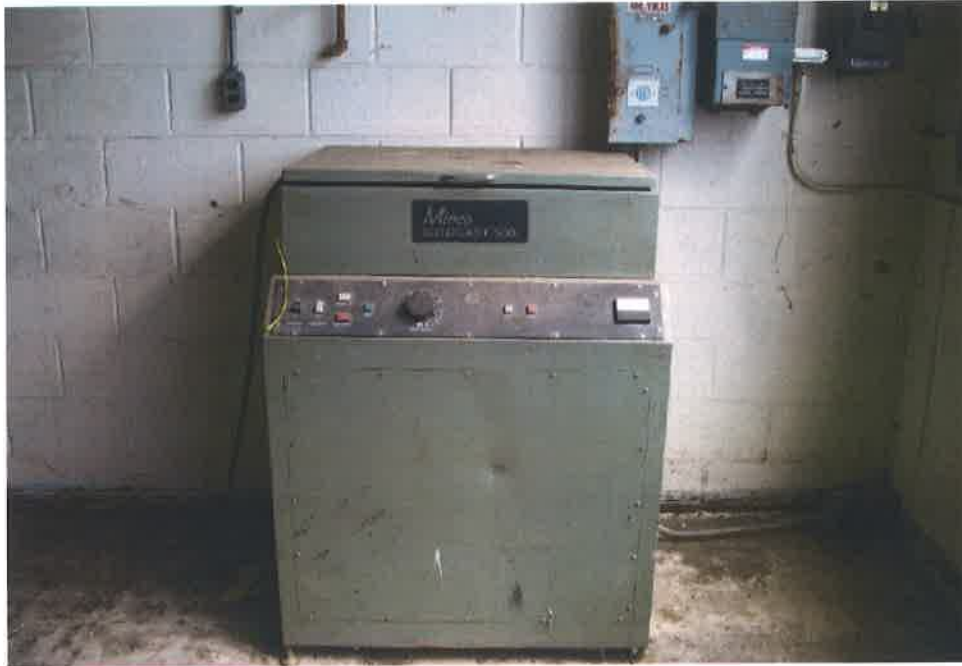
Equipment and electrical power supplies, SE corner of lab, SW corner of Service Building (9/27/2005)
