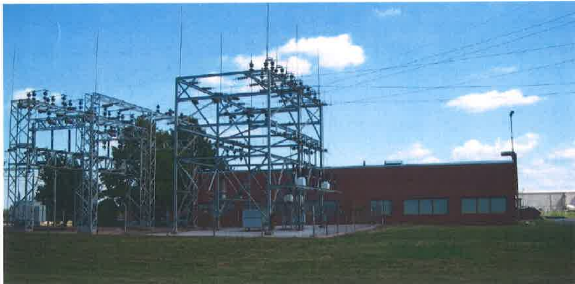
West end of Service Building, showing exhaust vent, with electrical substation in foreground (9/27/2005)
