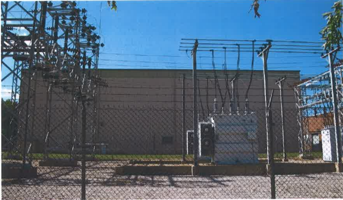
East end, Electron Beam Building with Electrical Substation in foreground (9/27/2005)
