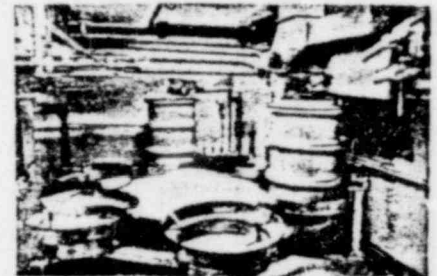
1,300 MWe PWR UNTERWESER, WEST GERMANY
