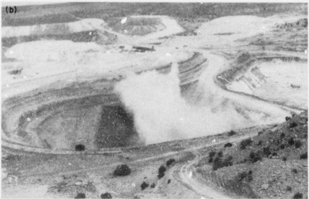
Figure 10. Sequential Pictures of Smoke and Dust from Blasting (time elapsed, approximately 3-4 minutes).
