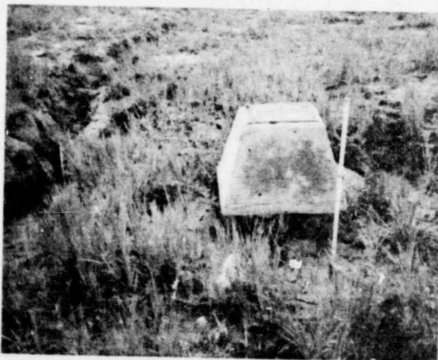
FIGURE 34: Erosion at Trench 24 west monument.
