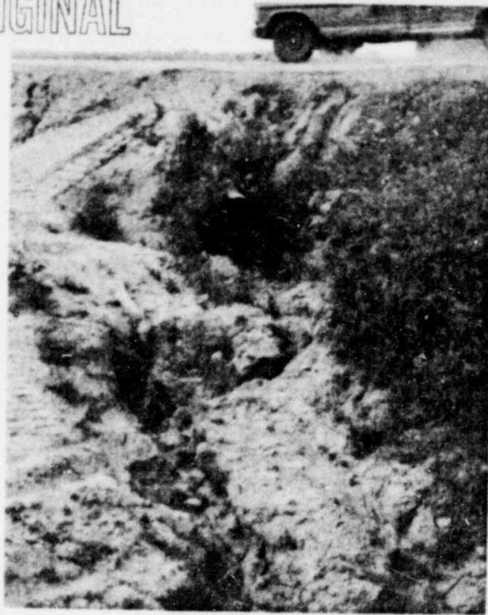
FIGURE 46: Roadway culvert which forms the head of DC-1; looking northwest beyond the northwest fence corner.
