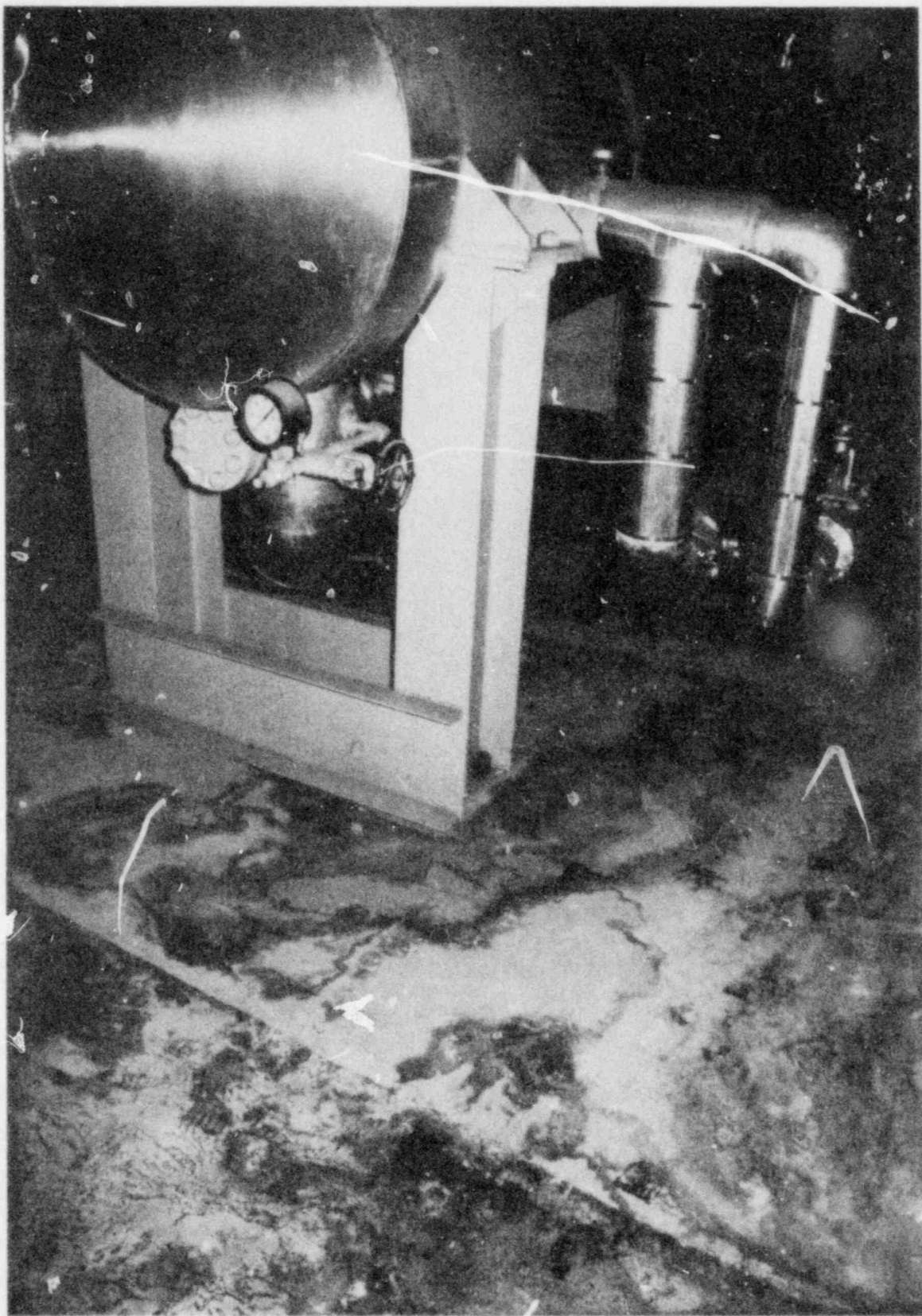
35 High-pressure feedwater heater anchorage
