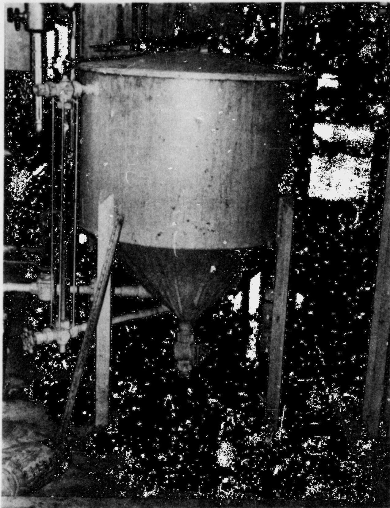
22 Pre-boiler chemical feed tank
