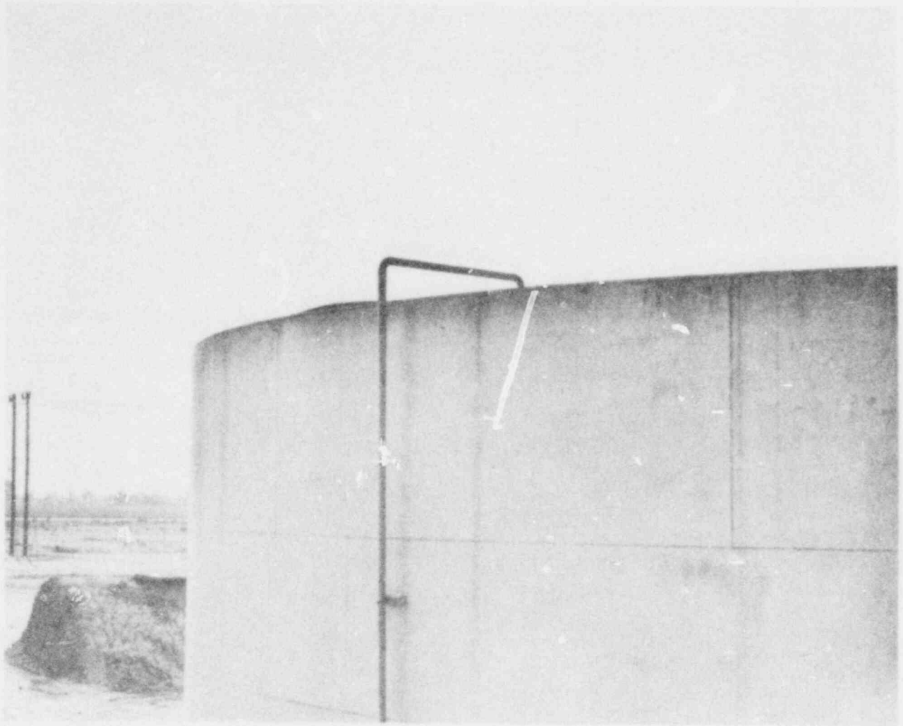
Fig. 13. Tank No. 3 was drained and entry was made during the August site visit. Of the 5 columns supporting the roof, one was badly buckled, causing the roof to sag locally. At about 90^{\circ} from the buckled column, the roof-to-tank wall weld joint had failed, opening up a crack several feet long where fuel oil sloshed out.
