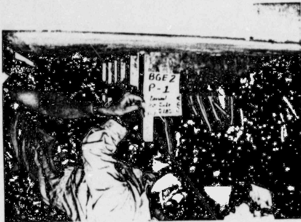
Figure II-3. Typical Kaowool Installation, Exposed Side
