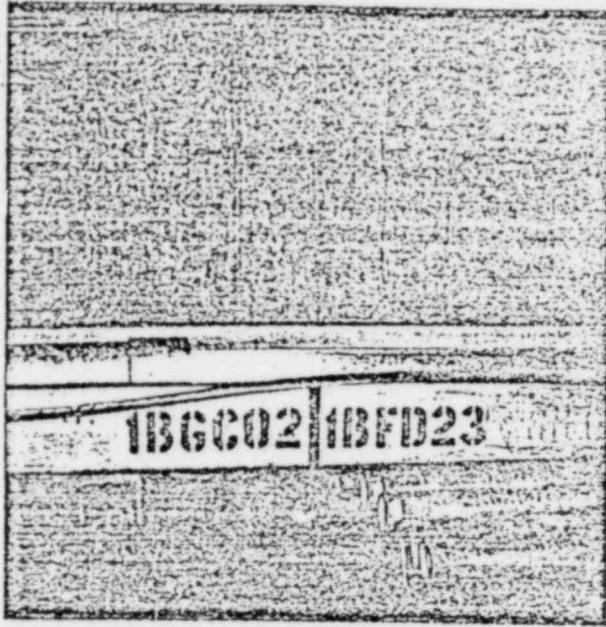
Fig 1. Upper Cable Spreading Room. Note: Identification is side by side as shown at beginning of each tray section. This tray is near a wall and the opposite side is inaccessible.
