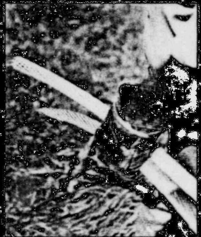
The diameter of this 250,000 KV conductor is nearly one inch. There's approximately 100 strands of high-tensile steel in the center of the conductor.
