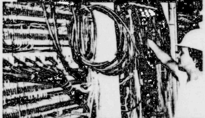
The complicated lines of electrical lines are made up of many different types of conductors and insulators.
