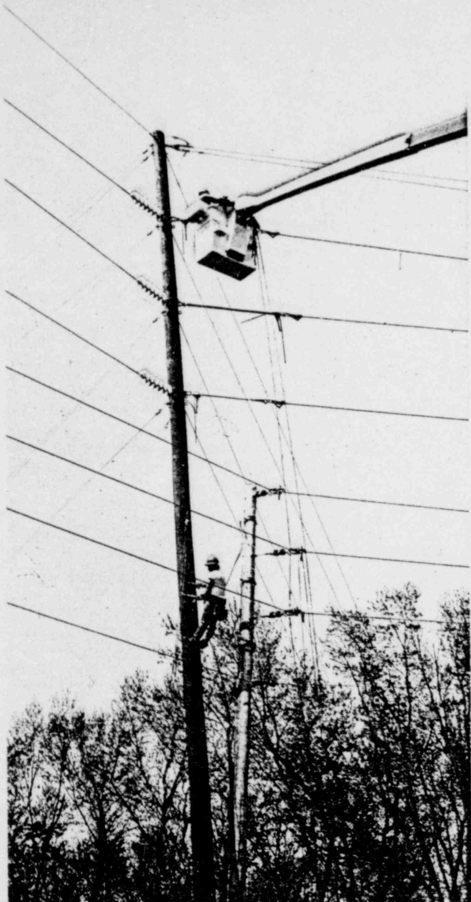
Dairyland Power Construction crews work on the four-mile N-149 line (69 kV Albion Tap off a Northern States Power Co. line) in Wisconsin near Black River Falls. This line was energized June 28, 1979.
