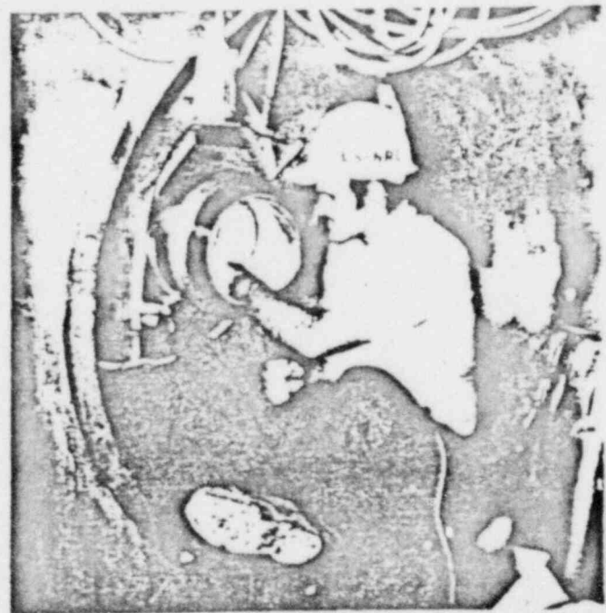
NRC resident inspector checks a weld in a reactor vessel thermal sleeve at the Susquehanna Steam Electric Station at Berwick, PA.
