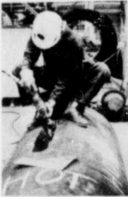
(c) GRINDING TO REMOVE FLAME EFFECTS
