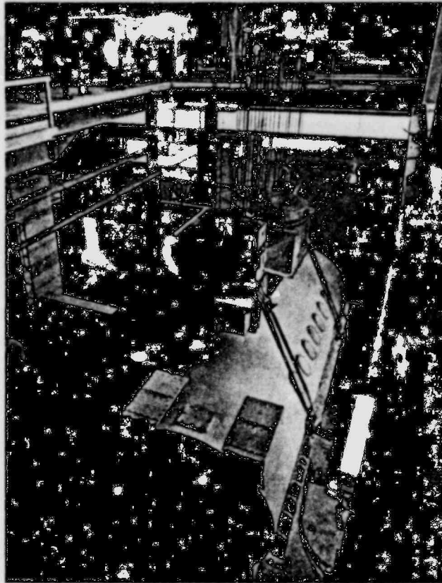
Lifting the stator (or housing) of the new generator at the Robert E. Ritchie Steam Electric Station in December was equivalent to lifting the weight of two fully-loaded Boeing 707 jet transports.
