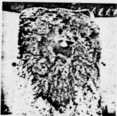
FIGURE 15. A 3-inch hole cut through 30-inch thick concrete slab.
