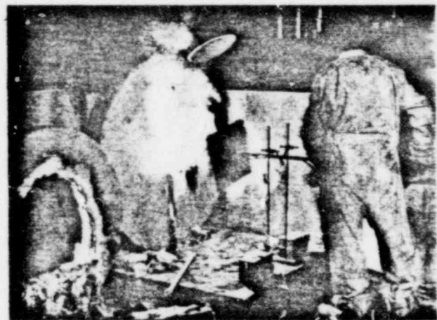
FIGURE 13. The first hole cut through concrete slab using early model of oxy-aluminum torch. Diameter of hole about 2 feet.
