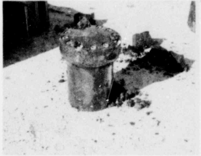
Figure 2.5.1.7-6. TB-1 Removed From AQ-1
