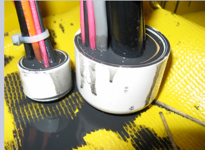
Sealed Cable Penetrant
