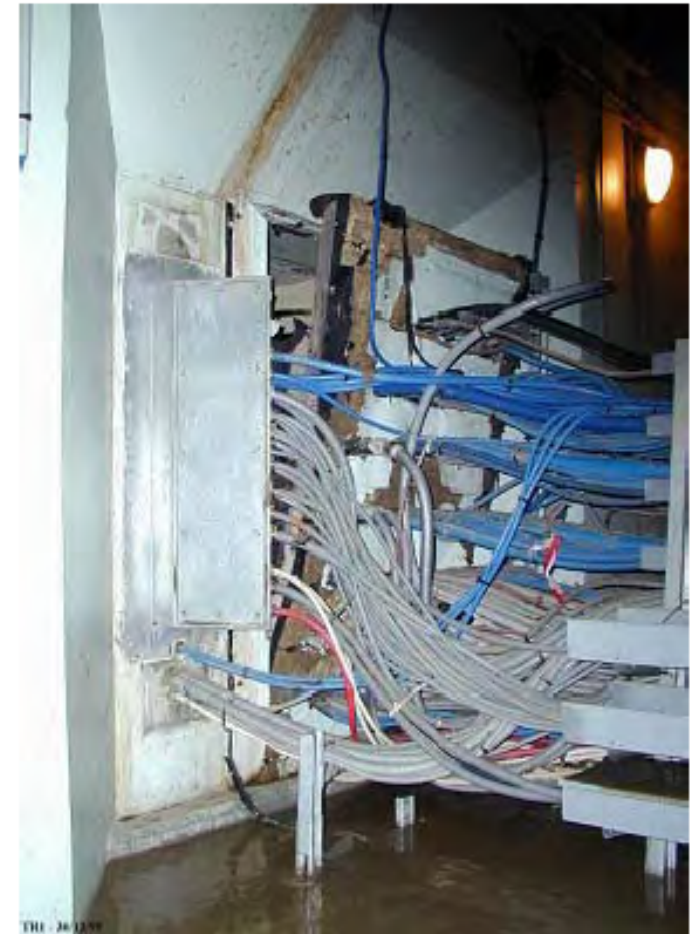
Failure of Cable opening
