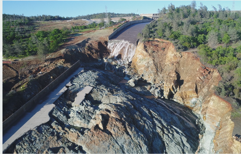
Oroville Dam, Feather River, Oroville, CA 770 feet (tallest embankment dam in US) Spillway Failure February 2017
