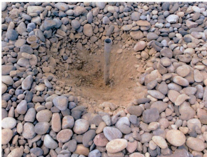
Photograph 9. Location 206 Riprap Dug Out
