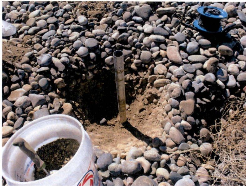
Photograph 11. Location 208 Riprap Dug Out
