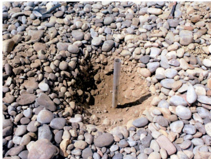
Photograph 8. Location 208 Riprap Dug Out
