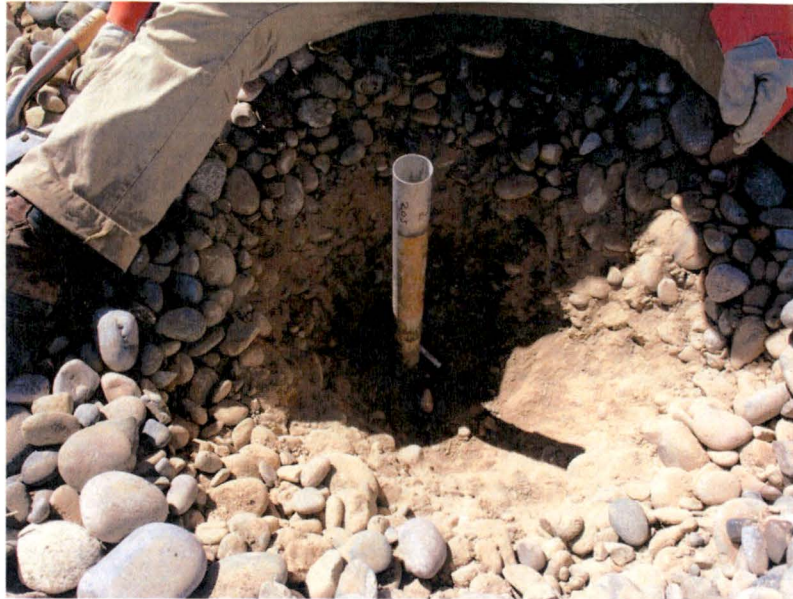
Photograph 10. Location 207 Riprap Dug Out
