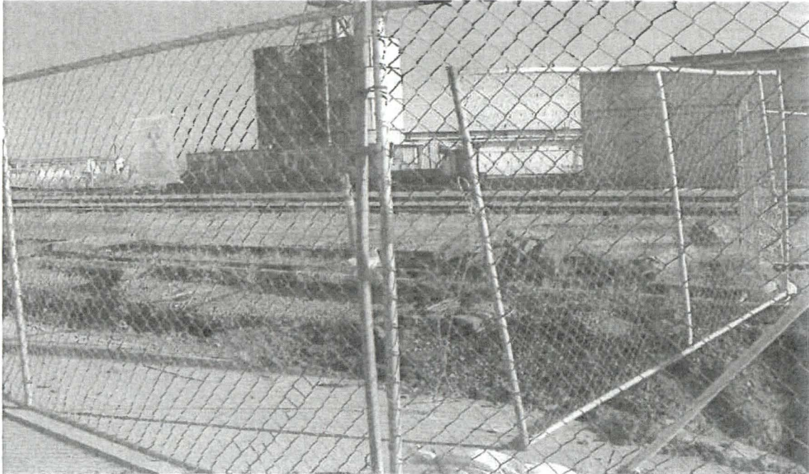
HPS: Inside "Utility Corridor (UC) Parcel" Active Construction Area (View B): RAD deficiency (uncollected/unused RAD rope strewn along fence panel) as noted/collected during end-of-day RAD integrity field check, 5.14.10
