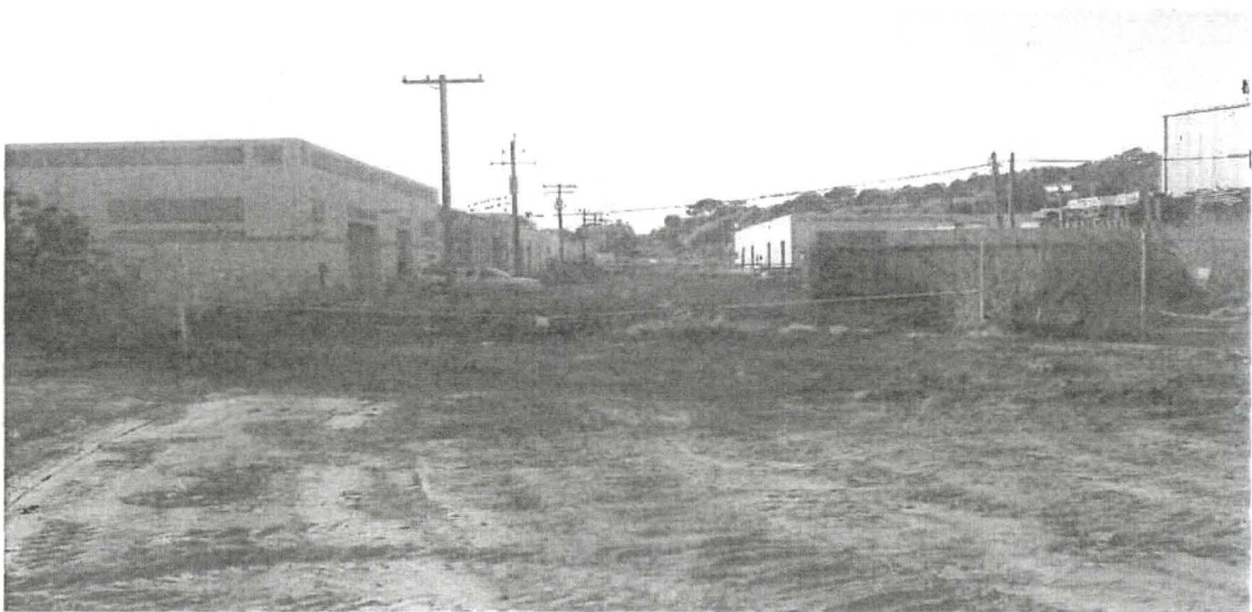
HPS Parcel E Site Perimeter: "Corrective Action" RCA Posting Established by RSO Representative during End of Day "RAD Integrity Field Check" at Construction Site referred to as "UCSF Access Road Detour" (Inside Site RCA Facing General Public Properties), Angle 1, March 18, 2010
