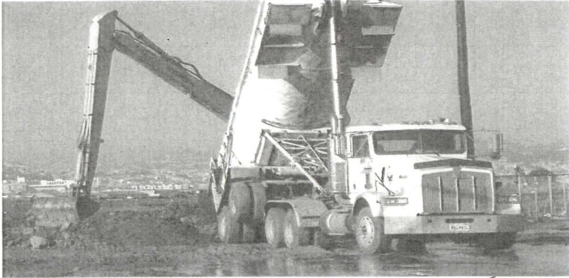
HPS Parcel E "Non-Impacted" Throughway: "As Found" by TtEQ RSO Representative after receipt of field call concerning Shaw's "IR-02" Construction Site and the staging of "clean" import fill inside established RCA (no RAD technician present to control work / monitor equipment going in/out of RCA), Shaw RSO Representative notified / corrective actions instituted; Angle 3, December 1, 2010
