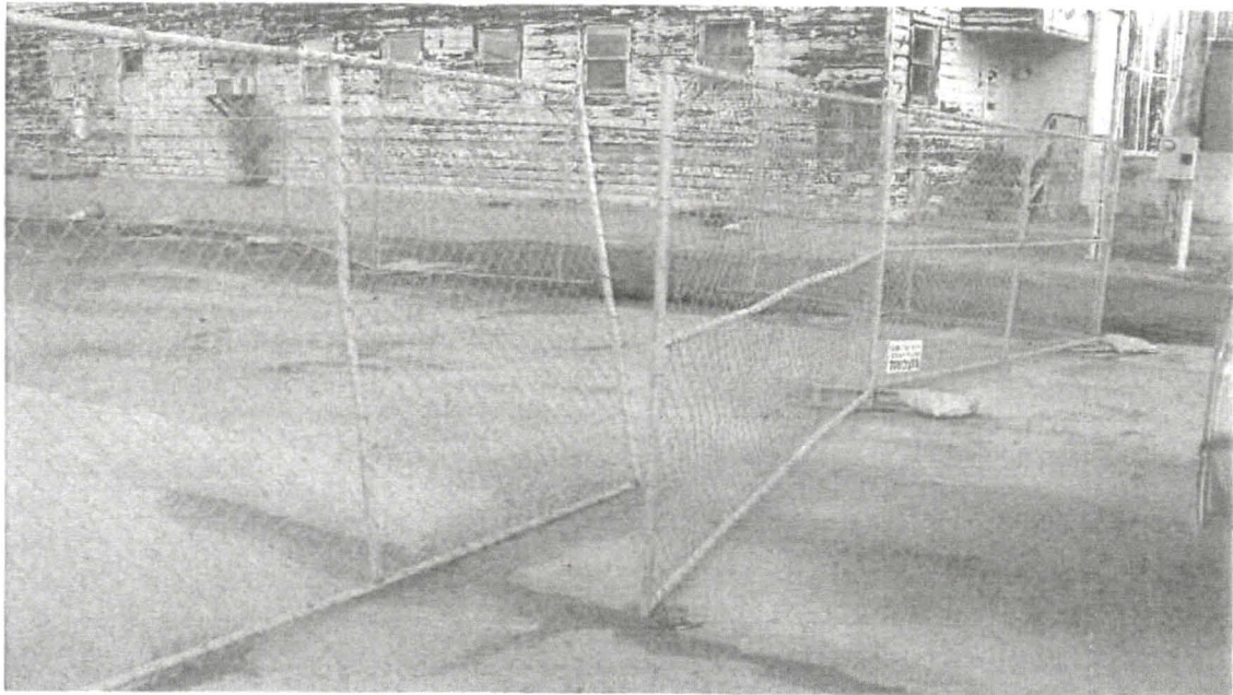
HPS Access to Utility Corridor (UC) Parcel: Active Construction Work Area: Safety deficiency (pad lock unsecured) as noted/corrected during end-of-day RAD integrity field check, 12.20.10
