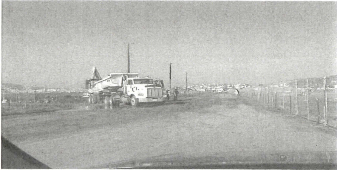
HPS Parcel E "Non-Impacted" Throughway: "As Found" by TTEC RSO Representative after receipt of field call concerning Shaw's "IR-02" Construction Site and the staging of "clean" import fill inside established RCA (no RAD technician present to control work / monitor equipment going in/out of RCA), Shaw RSO Representative notified / corrective actions instituted; Angle 1, December 1, 2010
