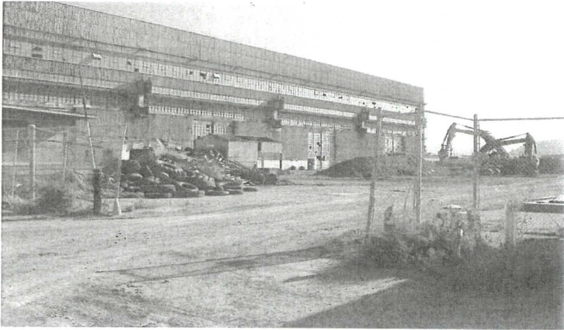
HPS Parcel D "Pickling Tank" Active Construction Area (View B): Safety deficiency as noted during end-of-day RAD integrity field check, 5.14.10
