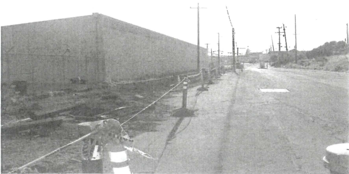
HPS: Inside "Utility Corridor (UC) Parcel" Active Construction Area (View D): Safety deficiency as corrected during end-of-day RAD integrity field check, 5.14.10
