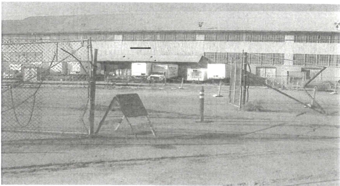
HPS: Entrance to "Utility Corridor (UC) Parcel" Active Construction Area (View A): Safety deficiency as corrected "Caution" tape re-established) during end-of-day RAD integrity field check, 5.14.10
