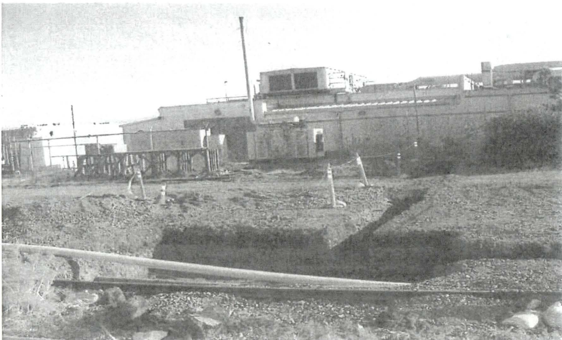
HPS: Inside to "Utility Corridor (UC) Parcel" Active Construction Area (View C): RAD deficiency (downed RAD rope) as noted/re-established during end-of-day RAD integrity field check, 5.14.10
