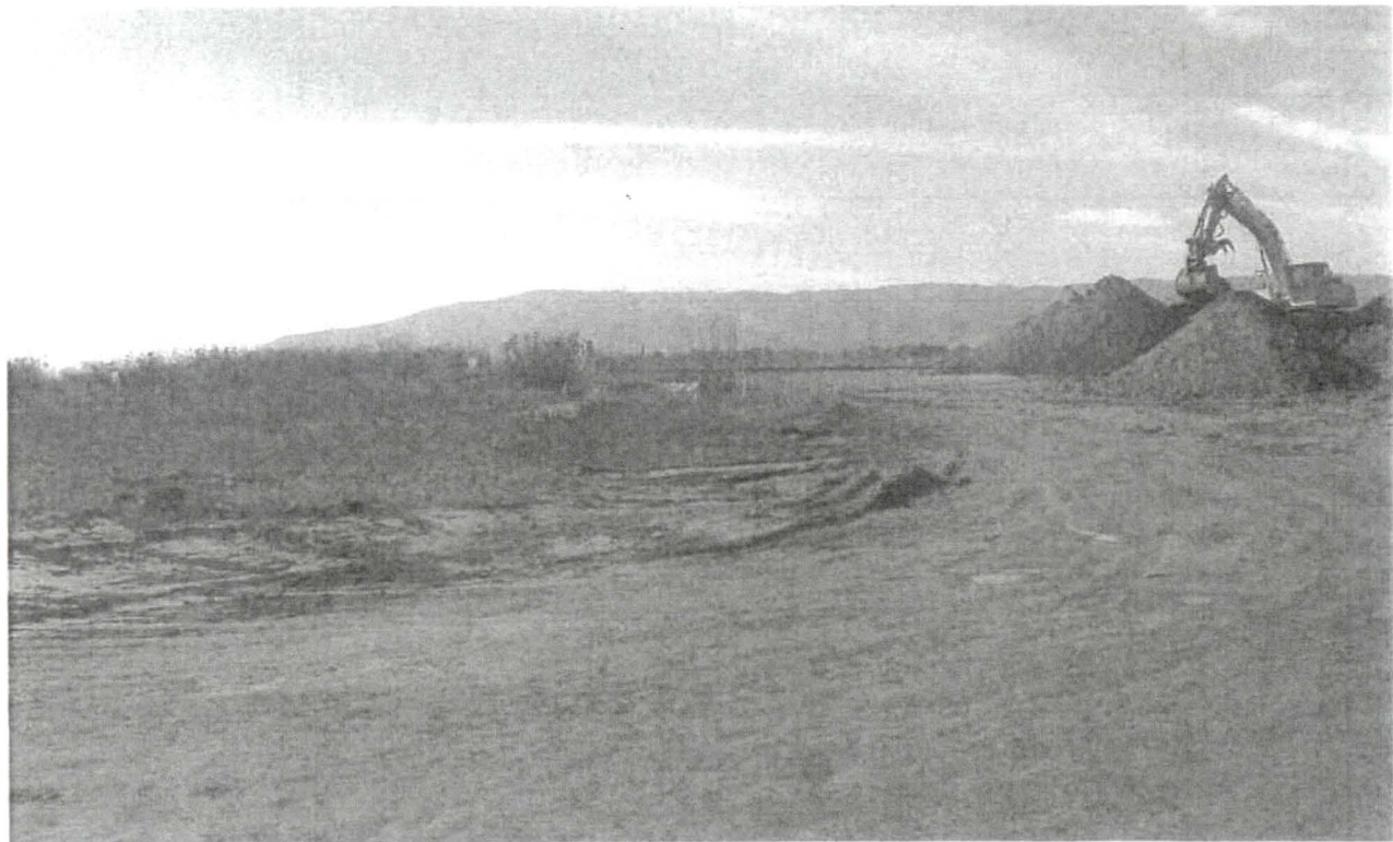
View 2 of 6: Parcel E Impacted Area "As Discovered" – Unauthorized Water Station Staged Inside RCA (w/ RAD Signage Compromise) 11.18.11
