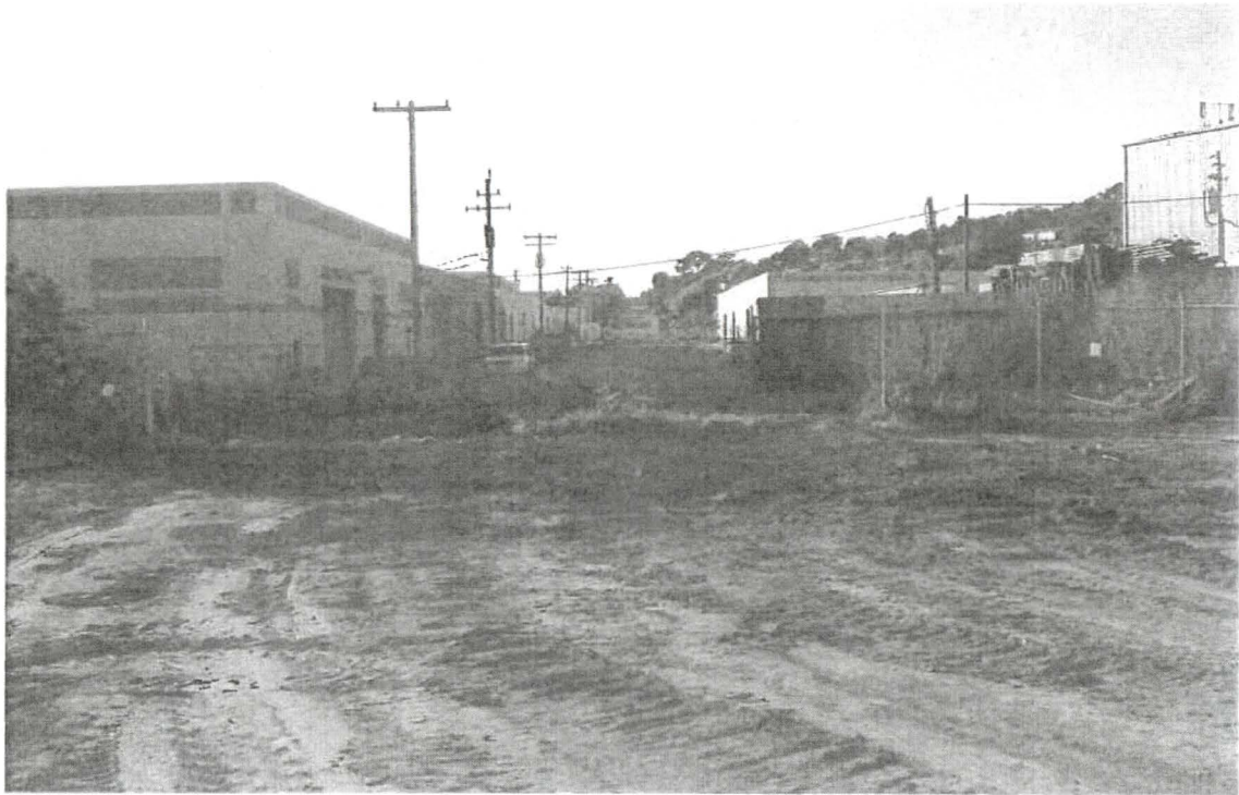
HPS Parcel E Site Perimeter: "As Found" by RSO Representative during End of Day "RAD Integrity Field Check" at Construction Site referred to as "UCSF Access Road Detour" (Inside Site RCA Facing General Public Properties), Angle 1, March 18, 2010
