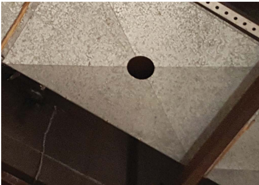
Photograph 23: Coupons were cut from HVAC ducts in Cell 6 to assess potential internal contamination.
