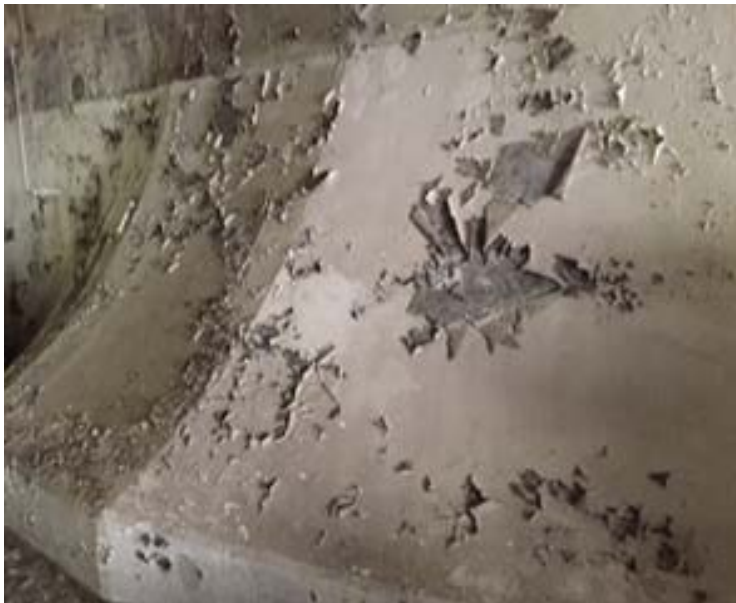
Photograph 3: Paint peeling on wall inside Cell 6 (typical of conditions observed in other cells of Building 181).
