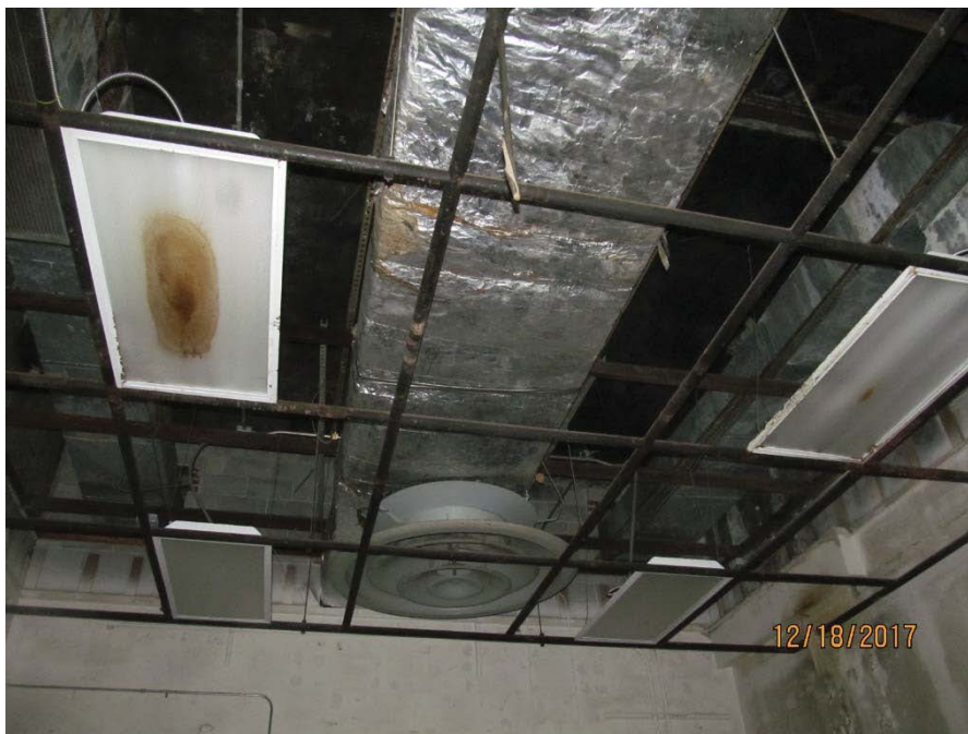
Photograph 7: Arrangement of HVAC supply and return in Room 6B1.
