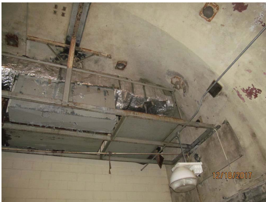
Photograph 8: HVAC at east end of Room 6A1.
