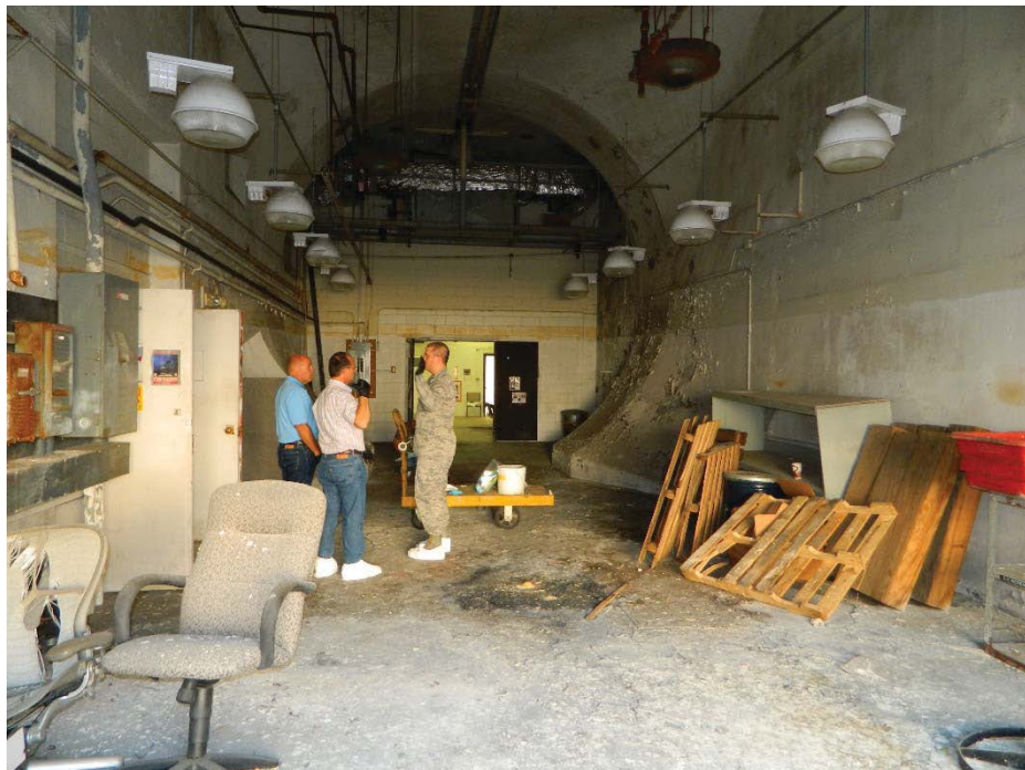
Photograph 2: Room 6A1 of Cell 6 looking east toward doorway into Room 6B1. Doorway to Room 3A on left side.
