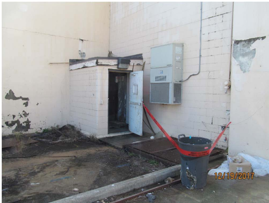
Photograph 25: East entrance to Room 6B1. Note, east exit of the pipe chase below the AC Unit.
