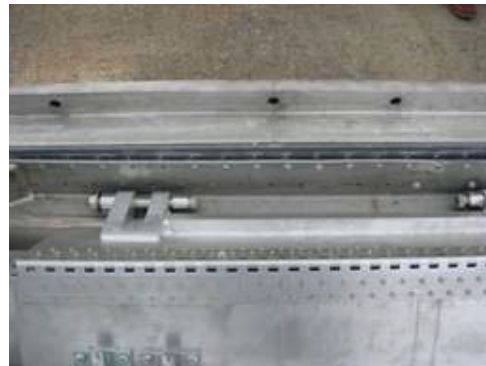
Figure 2-55 - Location of broken rivets
