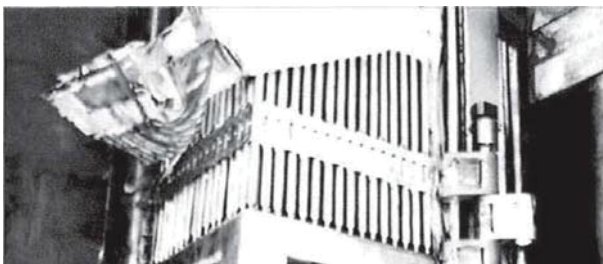
Figure 2-94 - Polypropylene sheet removal showing bright intact rods
