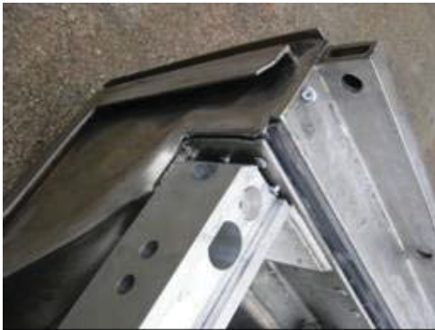
Figure 2-58 - Cracked top weld
