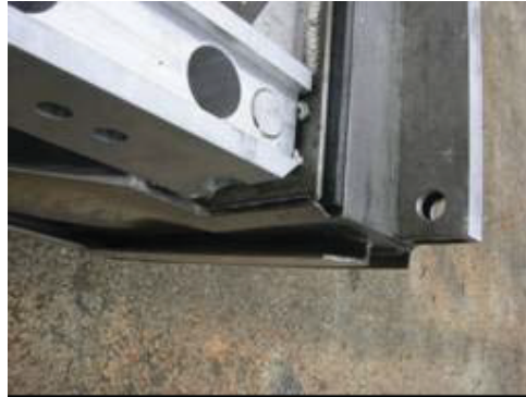
Figure 2-57 - Cracked top weld
